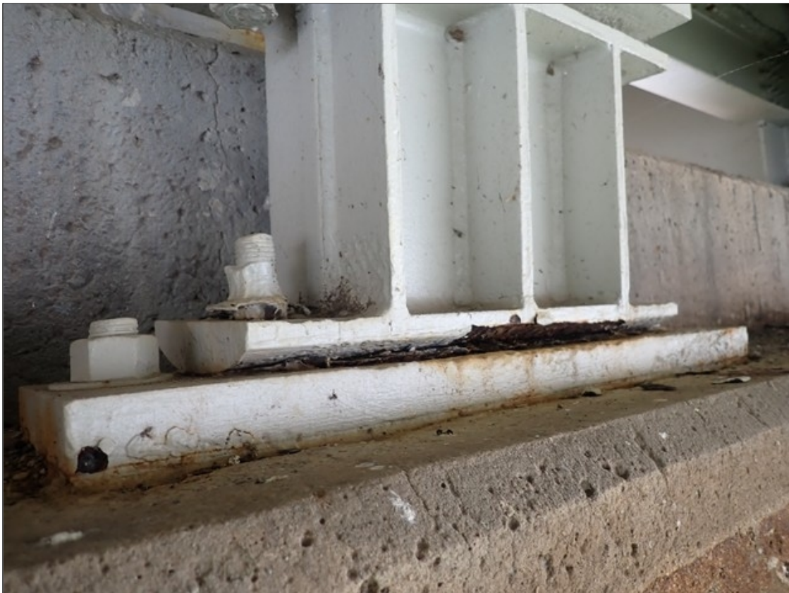
Span 2 Beam 3 Near Bearing: BEARING EXHIBITS PACK RUST [1/8 INCHES] WITH ACTIVE SURFACE CORROSION [NO SECTION LOSS NOTED] (CLEANED AND PAINTED) COATING UNDER ROCKER IS FAILING
