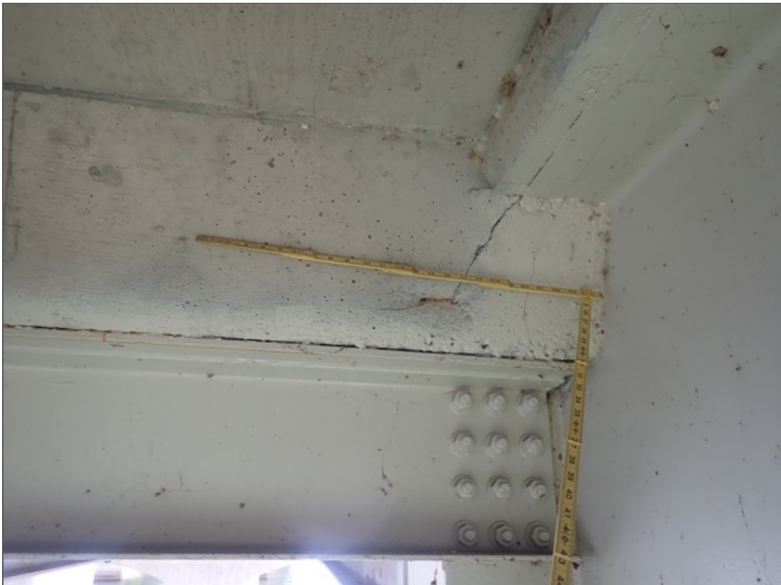
Span 9 Deck: DECK HAUNCH AT BEAM 1 OVER BENT 8, DELAMINATION/SPALL [18 INCHES LONG X 12 HIGH WIDE X 1-1/4 INCHES DEEP] WEST ONE [1] EXPOSED RUSTED REINFORCING [NO SECTION LOSS NOTED]
