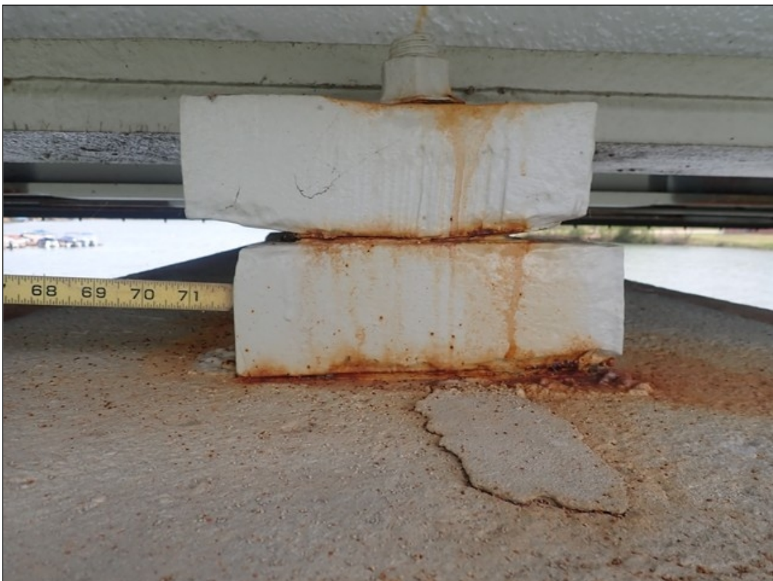
Span 6 Beam 1 Intermediate Bearing Bent 6: 1 1/8 INCHES CONTRACTION TO THE SOUTH
