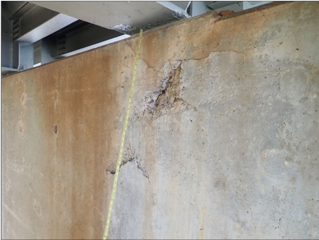
Bent 9 Cap 1: NORTH FACE UNDER BEAM 2, SPALL WITH EXPOSED REBAR AND AREA OF DELAMINATION [34 INCHES LONG X 32 INCHES HIGH X 1-1/2 INCHES DEEP]
