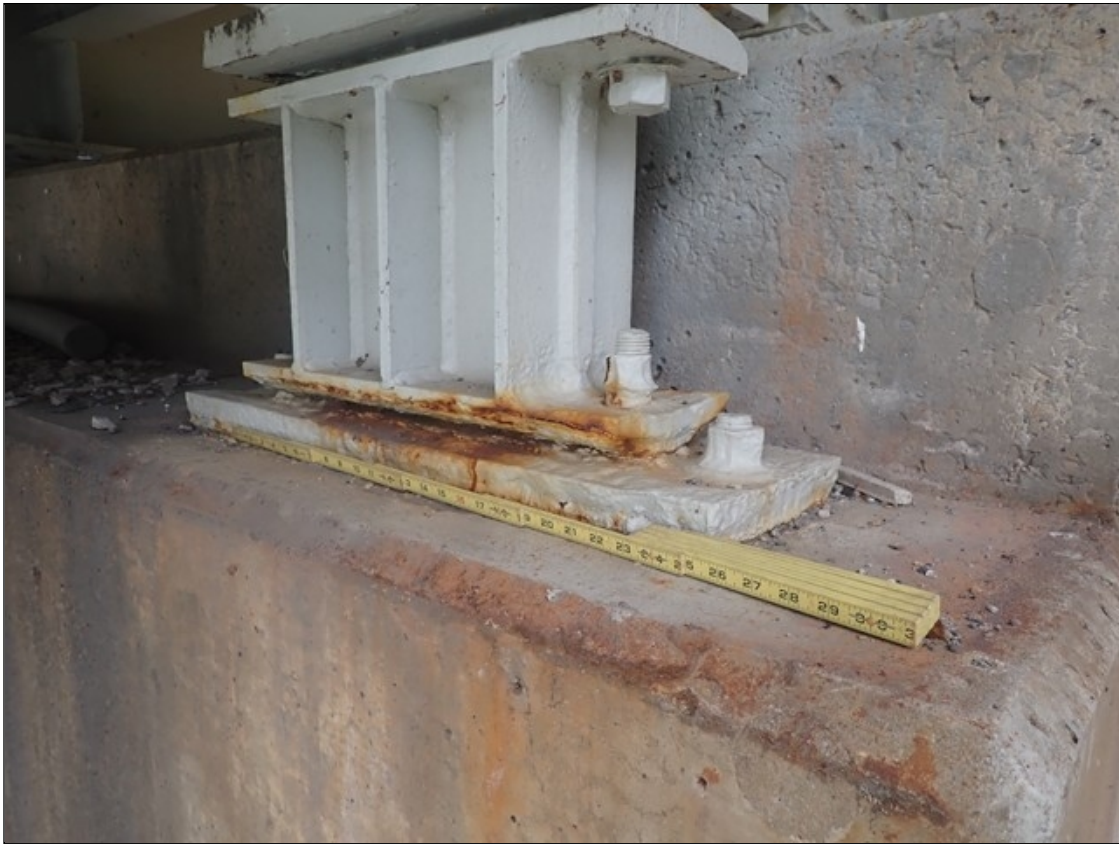
Span 6 Beam 4 Far Bearing: SURFACE RUST WITH PITTING
