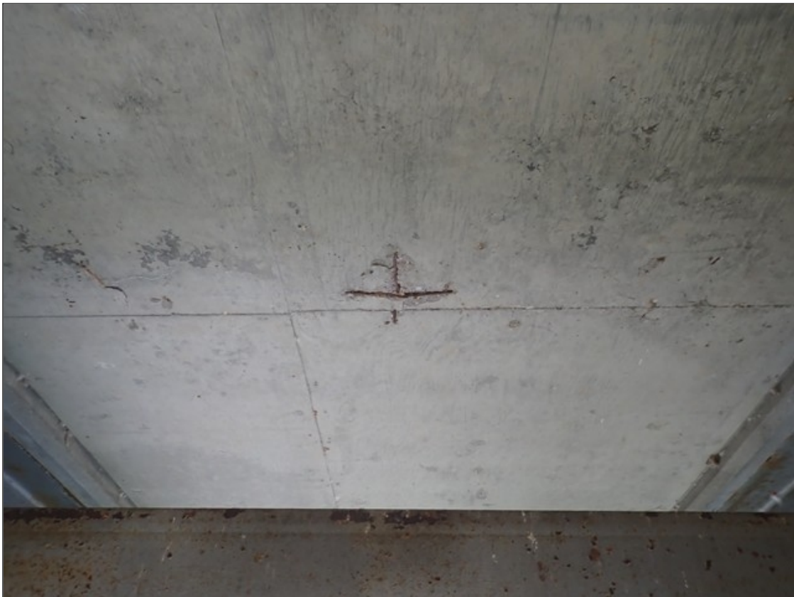
Span 9 Deck: 10 INCH LONG X 10 INCH WIDE X 1/2 INCH DEEP SPALL WITH EXPOSED REBAR CHAIRS ON BOTTOM OF DECK IN BAY 3 NEAR MIDSPAN
