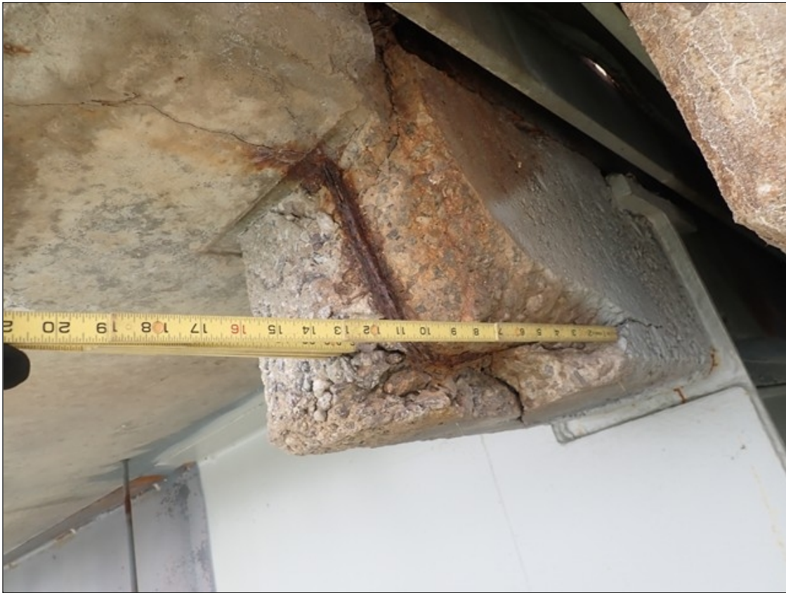
Span 6 Deck: 2 FEET WIDE X 8 INCH LONG X 12 INCH TALL SPALL WITH EXPOSED REBAR IN LEFT END DIAPHRAGM OVER BENT 5
