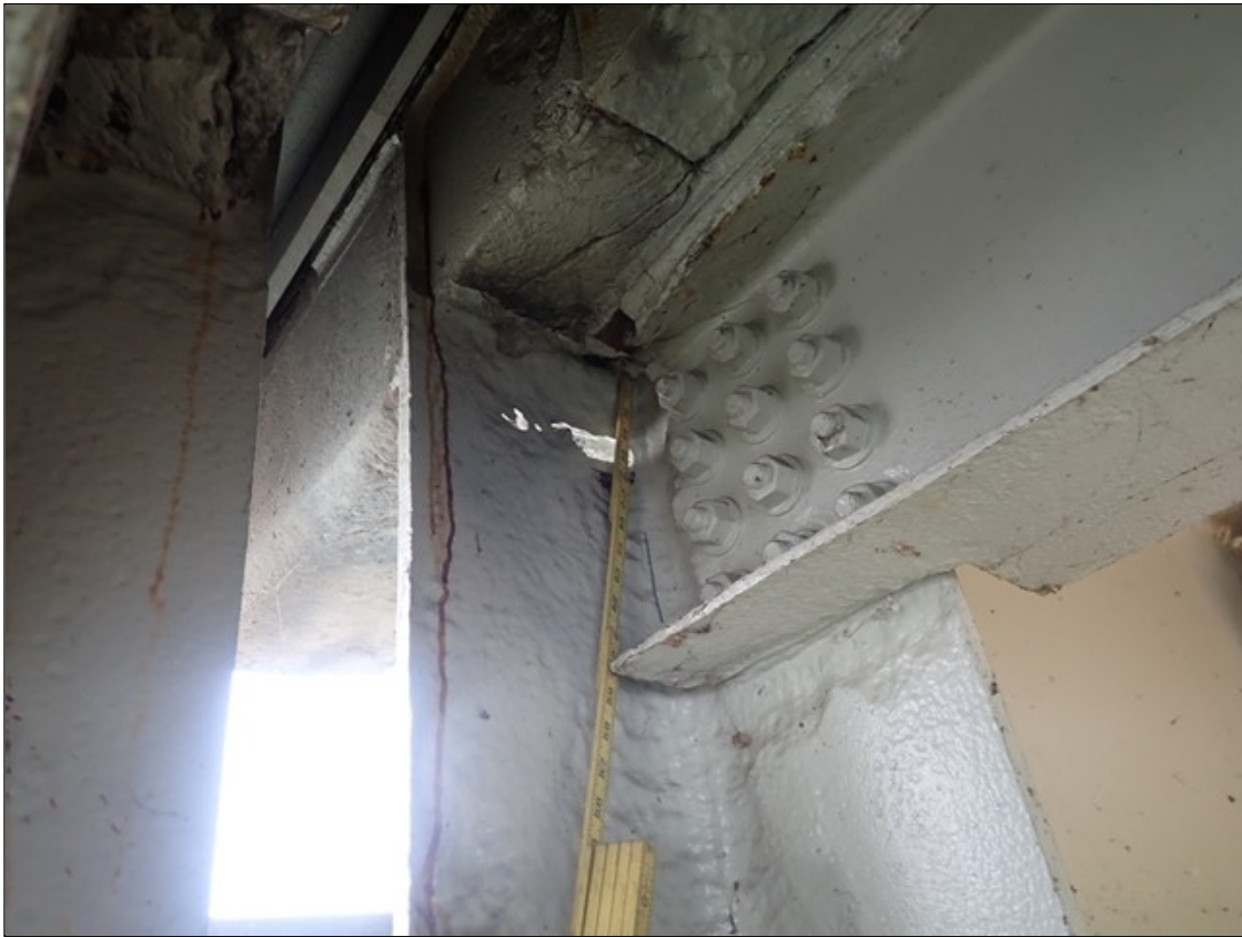
Span 10 Beam 1: AT NEAR END, CORROSION WITH SECTION LOSS, UPPER WEB AT DIAPHRAGM: CORROSION HOLE [6 INCHES LONG X 3 INCHES TALL AT 3 INCHES DOWN FROM DIAPHRAGM]; LOWER WEB: [9 INCH X 24 INCHES - AVERAGE REMAINING 7/16 INCHES]; BOTTOM FLANGE: [12 INCHES X FULL WIDTH - AVERAGE REMAINING 3/4 INCHES] (CLEANED AND PAINTED) (PAR)
