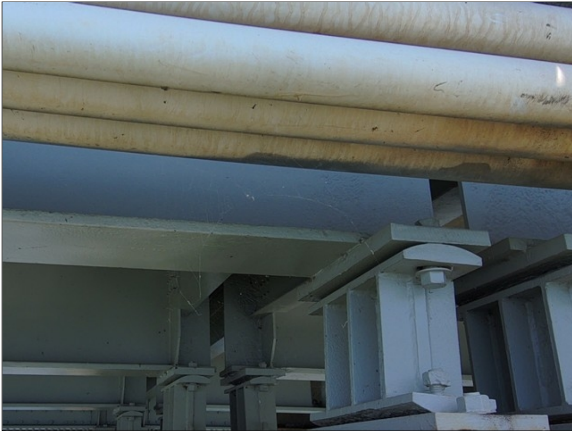
Span 6 Beam 1: NEAR END AT BENT 5, CORROSION WITH SECTION LOSS, LOWER WEB: [3 FEET LONG X 4 INCHES HIGH - AVERAGE REMAINING 3/8 INCHES] ; BOTTOM FLANGE: [18 INCHES LONG X FULL WIDTH - SECTION LOSS LESS THAN 1/16 INCHES] (UPPER WEB REPAIRED IN 2022) (PAR)
