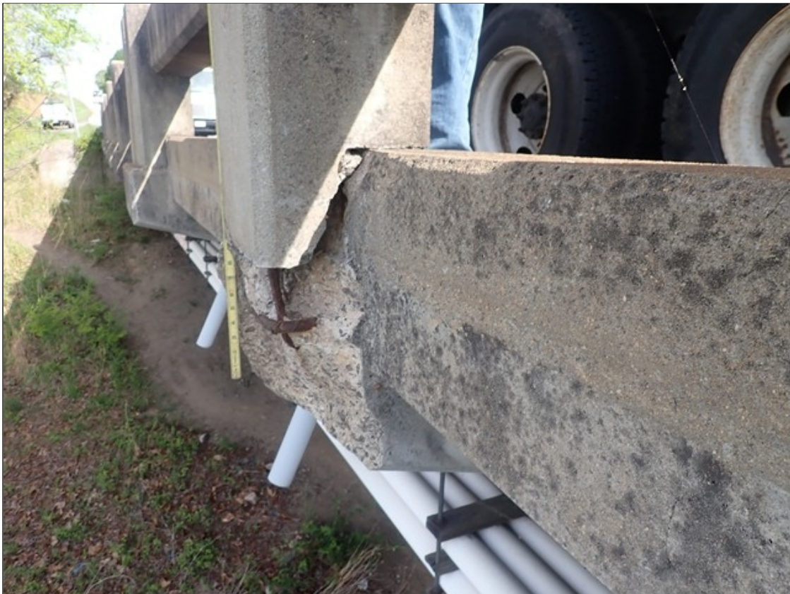
Span 10 Left Bridge Rail: 14 INCHES LONG X 17 INCHES HIGH X 9 INCHES DEEP SPALL WITH EXPOSED REBAR ON OUTSIDE FACE OF POST 5 (PAR)
