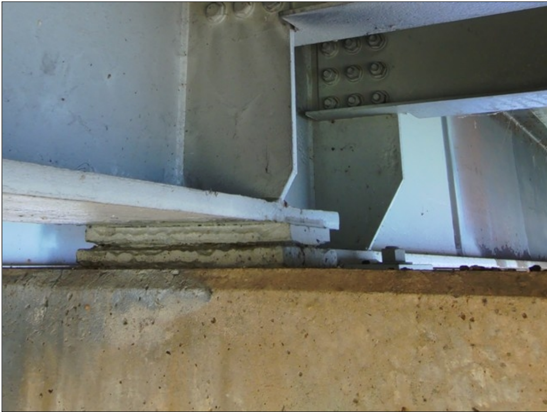
Span 10 Beam 3: [PAR] AT NEAR END, CORROSION WITH SECTION LOSS, WEB OVER BEARING: [23 INCHES LONG X UP TO FULL HEIGHT - AVERAGE REMAINING 1/2 INCHES]; BOTTOM FLANGE: [14 INCHES LONG X FULL WIDTH - AVERAGE REMAINING 1-1/8 INCHES] (CLEANED AND PAINTED)
