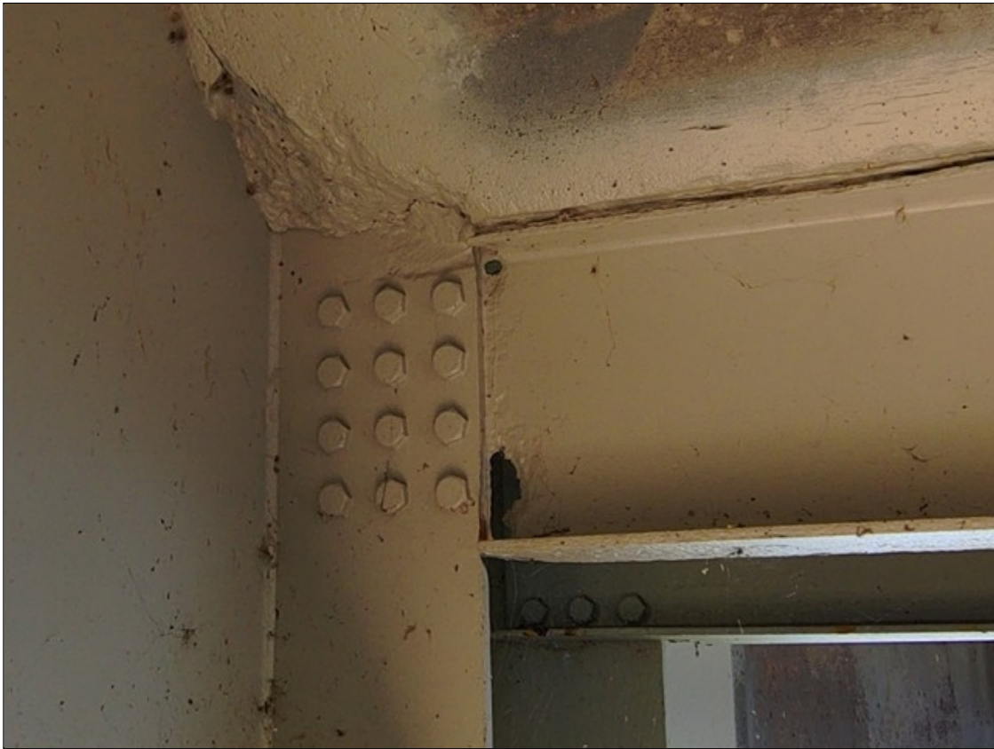
AT END DIAPHRAGM IN BAY 1 ADJACENT TO BEAM 1, ACTIVE CORROSION WITH SECTION LOSS [AVERAGE LOSS OF 1/8 INCH WITH 3 INCH LONG X 1 INCH HIGH CORROSION HOLE] (CLEANED AND PAINTED); TEMPORARY REPAIR: 5 FEET LONG X 21 INCHES HIGH WELDED REPAIR TO WEB AT BENT 1 (PAR)
