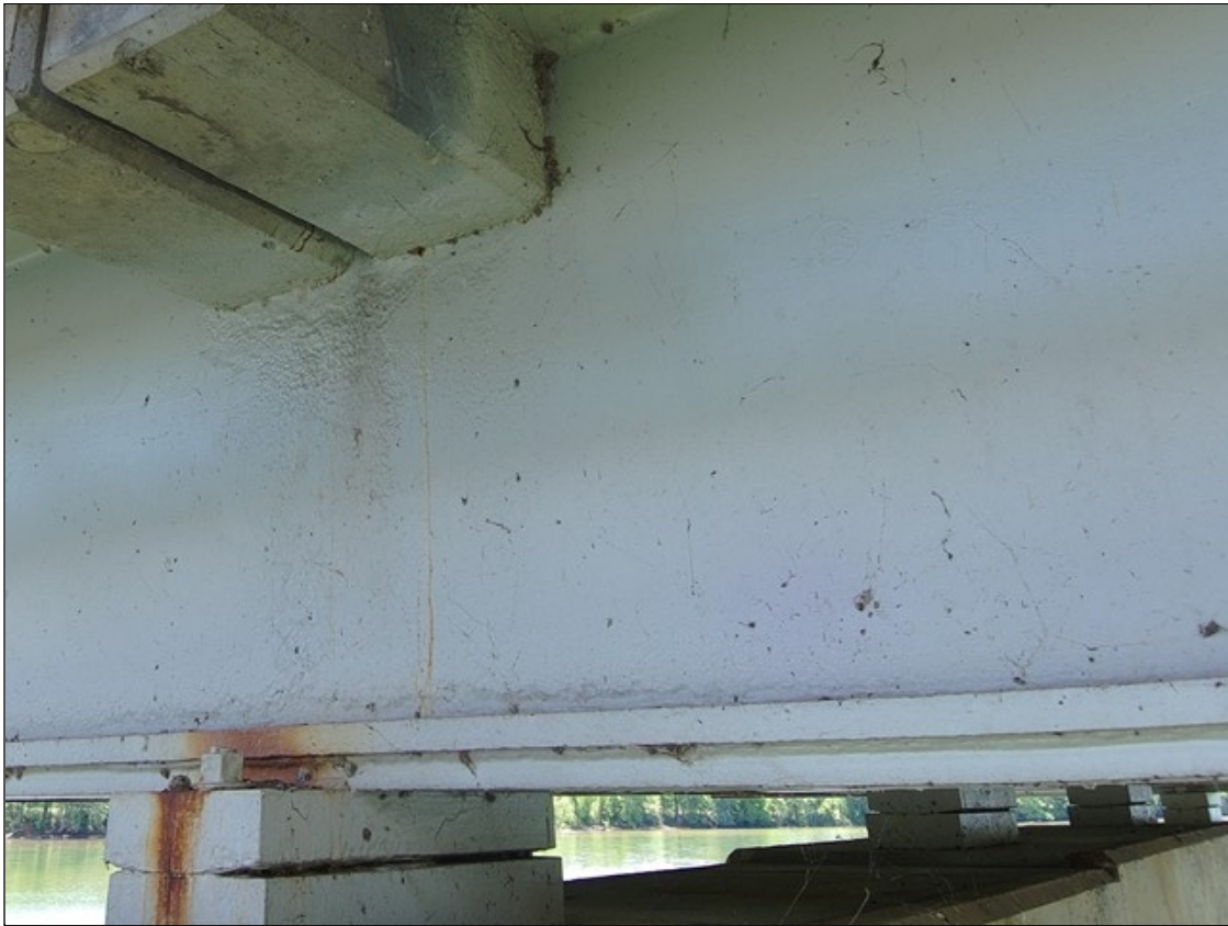
Span 6 Beam 4: OVER BENT 8 UPPER WEB AT DIAPHRAGM, CORROSION [24 INCHES LONG X UP TO 3 INCHES HIGH - AVERAGE REMAINING 5/8 INCHES]; LOWER WEB [4 FEET LONG X 2 INCHES WIDE - AVERAGE REMAINING 5/8 INCHES] (PAINTED WITH NO RUST) (PAR)
