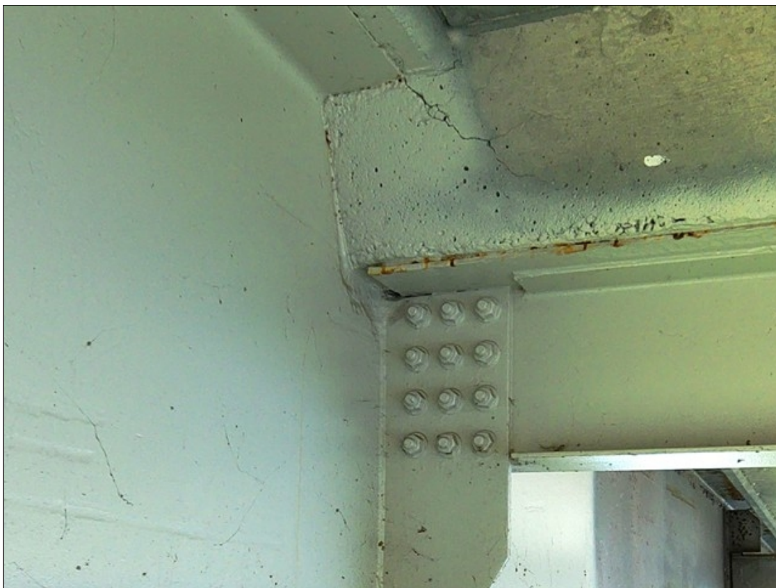
Span 2 Beam 3: OVER BENT 2, CORROSION WITH SECTION LOSS UPPER WEB ADJACENT TO DECK HAUNCH: [22 INCHES LONG X UP TO 10 INCHES WIDE - AVERAGE REMAINING 5/16 INCHES] (CLEANED AND PAINTED) (PAR)
