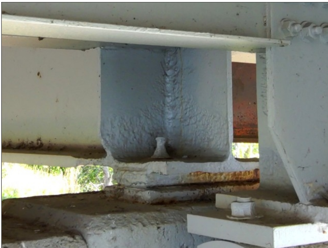
Span 1 Beam 3: 9 INCH LONG X 9 INCH HIGH AREA OF 1/8 INCH SECTION LOSS (3/8 INCH REMAINING) WITH NO RUST ON BOTH SIDES OF STIFFENER AT BENT 1 (CLEANED AND PAINTED) (PAR)
