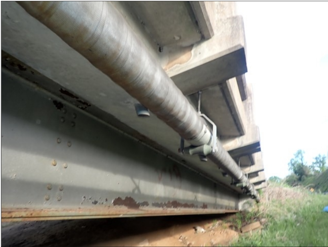
UTILITY EAST SIDE
