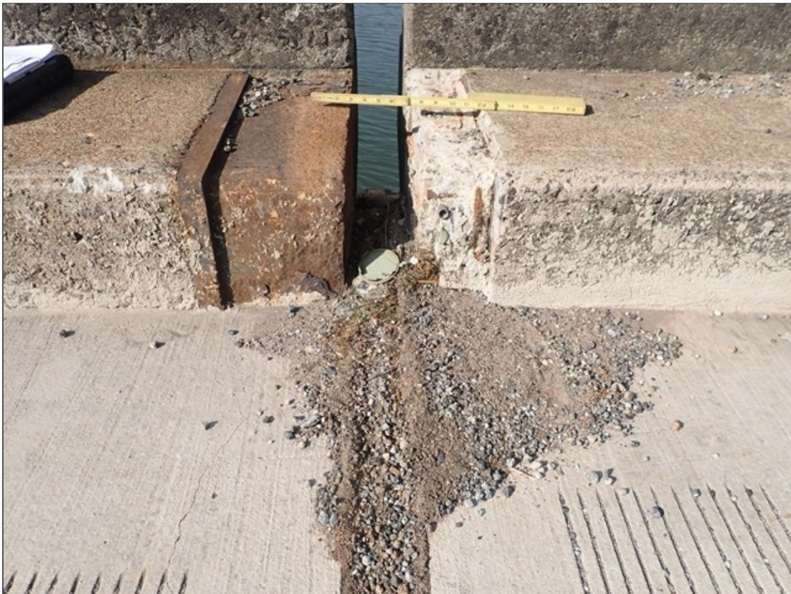
Span 10 Left Bridge Rail: STEEL COVER PLATE MISSING AT CURB
