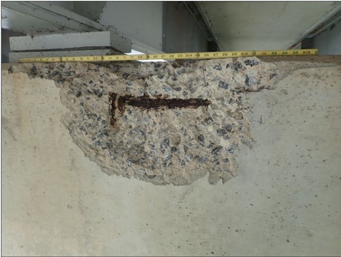
Bent 6 Cap 1: 36 INCHES LONG X 15 INCHES TALL X 6 INCHES WIDE SPALLING WITH EXPOSED REBAR WITH SECTION LOSS ON SOUTH FACE AND TOP OF CAP UNDER GIRDER 2 (PAR)
