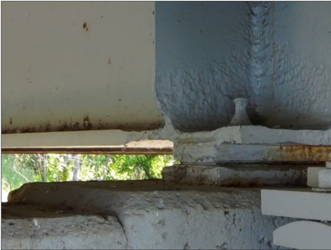
Span 1 Beam 3: FAR END, CORROSION WITH SECTION LOSS: BOTTOM FLANGE [15 INCHES LONG X FULL WIDTH - AVERAGE REMAINING 5/8 INCHES]; WEB OVER BEARING [9 INCHES LONG X FULL HEIGHT - AVERAGE REMAINING 1/2 INCHES] (CLEANED AND PAINTED) (PAR)
