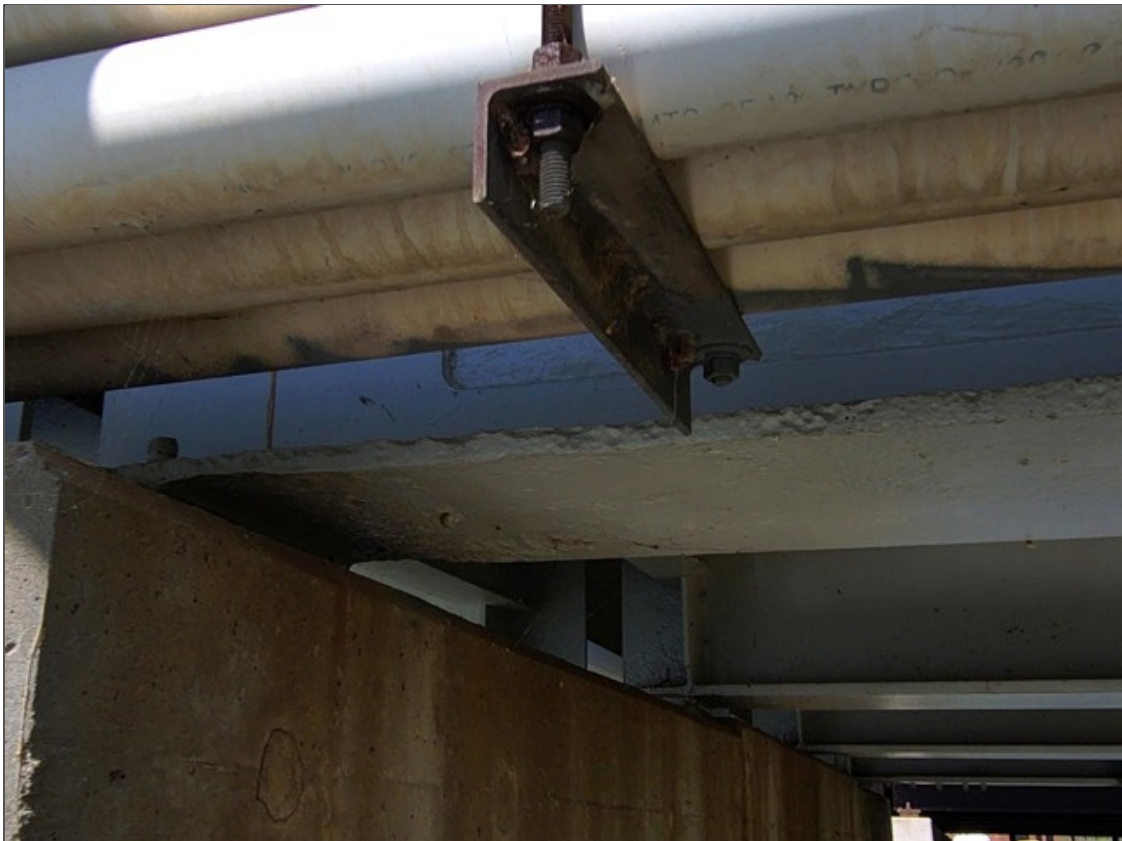
Span 1 Beam 1: AT FAR END, CORROSION WITH SECTION LOSS: BOTTOM FLANGE [18 INCHES LONG X FULL WIDTH - AVERAGE REMAINING 7/8 INCHES] (CLEANED AND PAINTED) (PAR)
