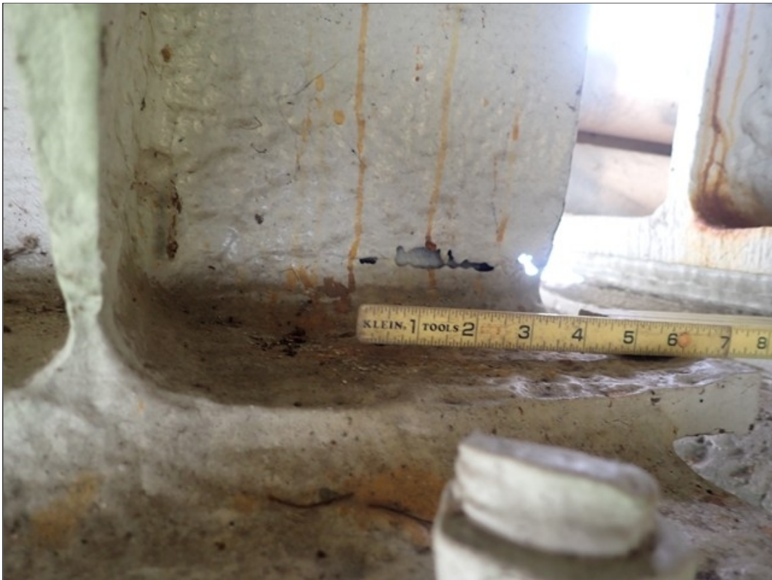
Span 6 Beam 1: IN SPAN 9 AT FAR END, CORROSION WITH SECTION LOSS, BOTTOM FLANGE: [15 INCHES LONG X FULL WIDTH - AVERAGE REMAINING 3/4 INCHES] (CLEANED AND PAINTED) (PAR)
