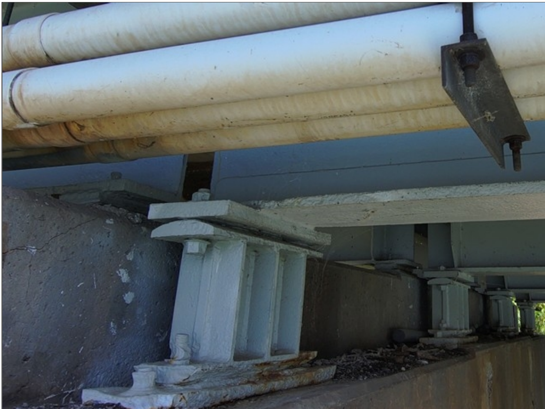
Span 6 Beam 1: [PAR] IN SPAN 9 AT FAR END, CORROSION WITH SECTION LOSS, BOTTOM FLANGE: [15 INCHES LONG X FULL WIDTH - AVERAGE REMAINING 3/4 INCHES] (CLEANED AND PAINTED)
