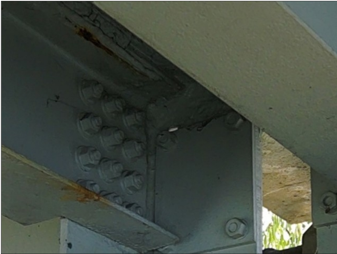
Span 10 Beam 4: PAR: 1 INCH DIAMETER AREA OF COMPLETE SECTION LOSS IN TOP OF WEB STARTING 6 INCHES FROM BEAM END AND 2 INCHES DOWN FROM DIAPHRAGM AT BENT 9 (CLEANED AND PAINTED)
