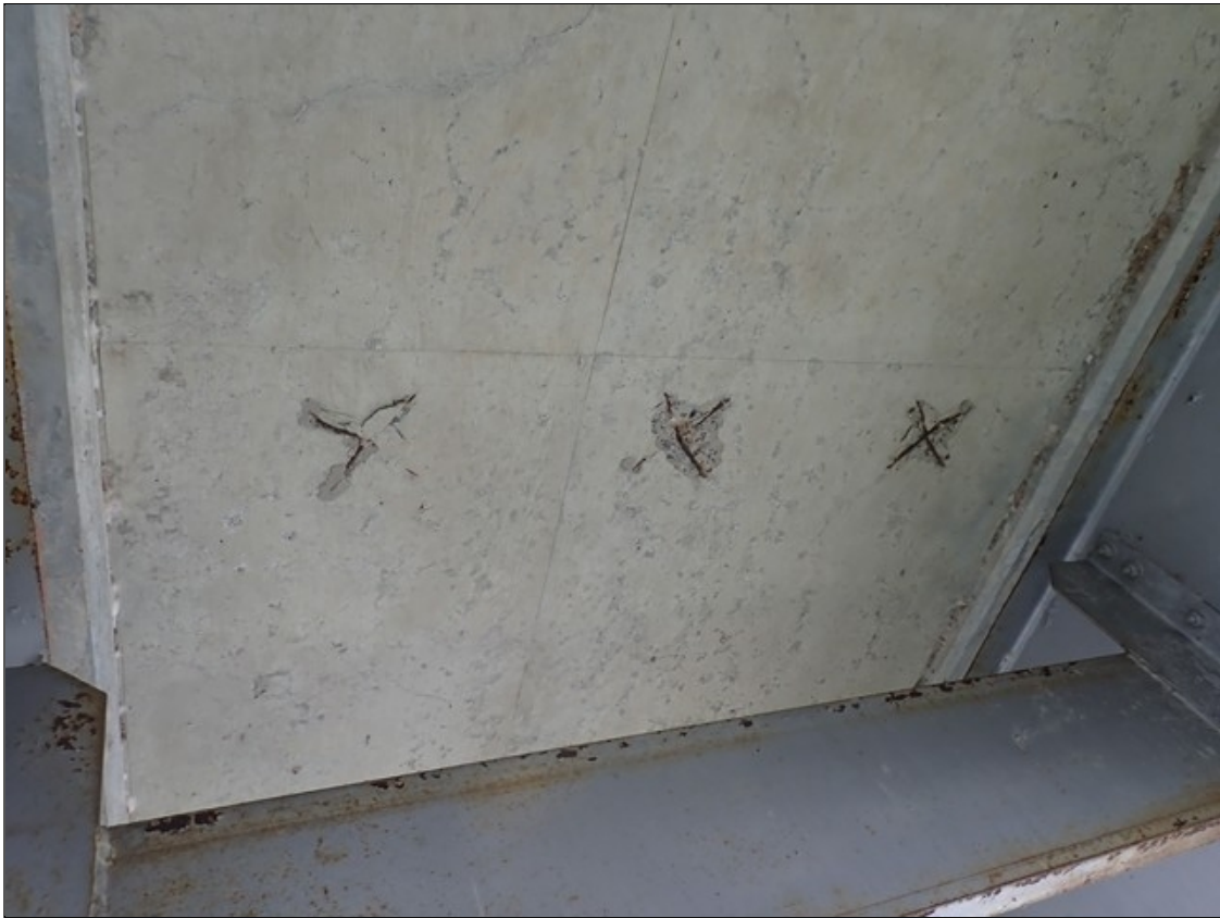
Span 7 Deck: (3) UP TO 9 INCH LONG X 9 INCH WIDE X 1/2 INCH DEEP SPALLS WITH EXPOSED REBAR ON BOTTOM OF DECK NEAR MIDSPAN AT RANDOM THROUGHOUT EACH BAY
