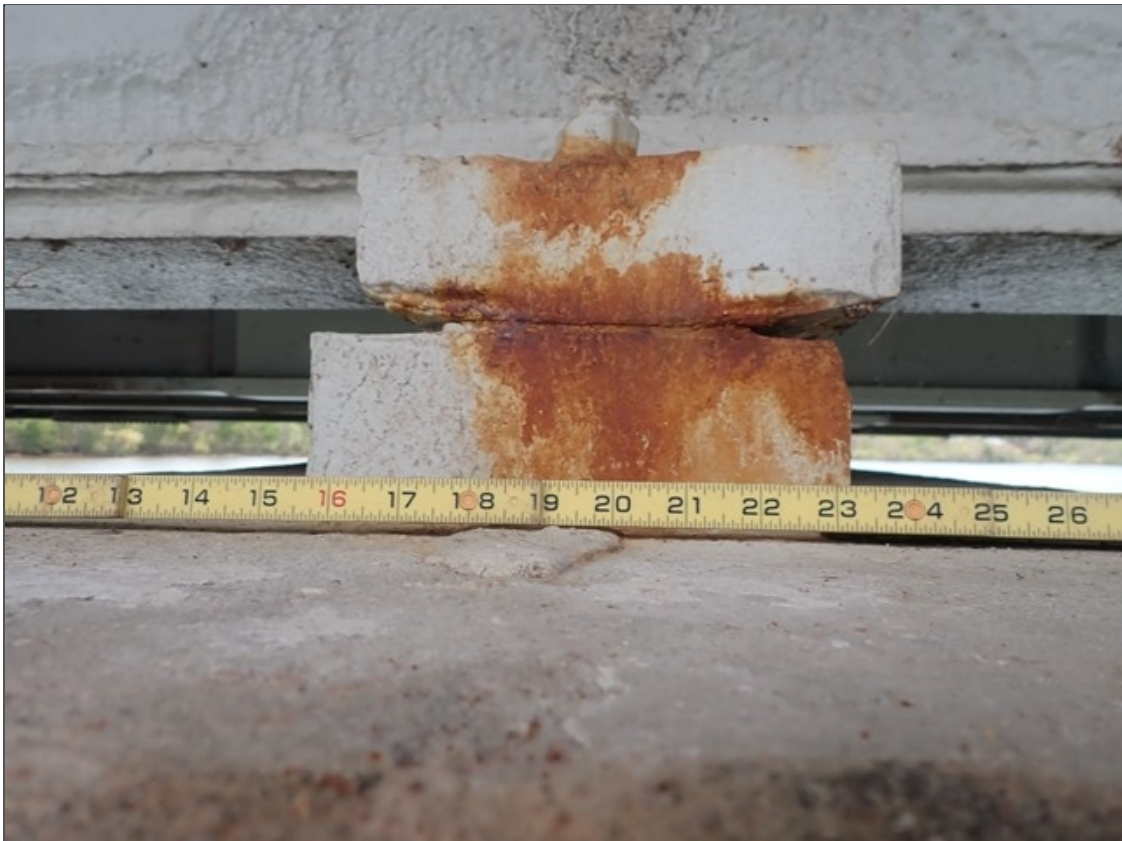
Span 6 Beam 4 Intermediate Bearing Bent 6: BEARING OVER BENT 6 EXHIBITS PACK RUST [1/8 INCHES] (CLEANED AND PAINTED)
