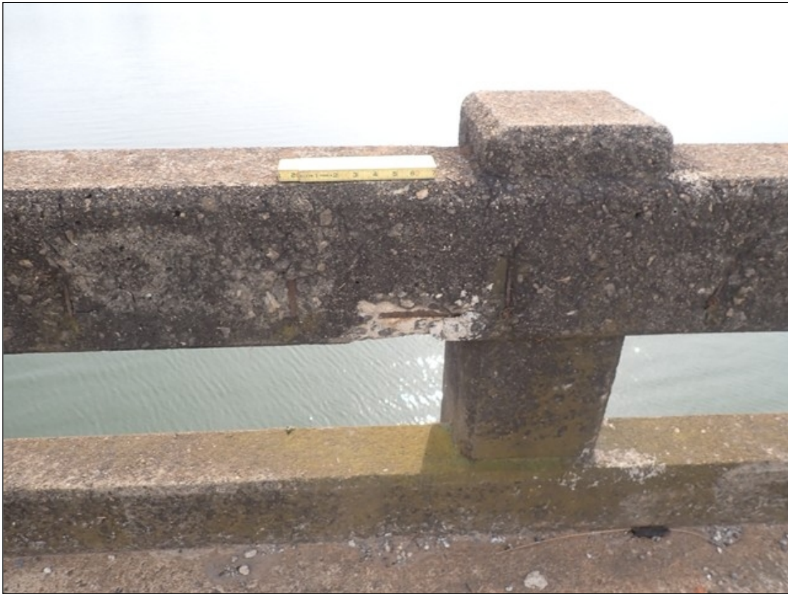
Span 7 Left Bridge Rail: (10) UP TO 8 INCHES LONG X 3 INCHES HIGH X 1 INCH DEEP SPALLS WITH EXPOSED REBAR ON RAIL BETWEEN POSTS 3 AND 6
