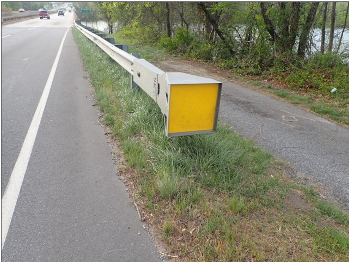
NORTHWEST GUARDRAIL TERMINAL
