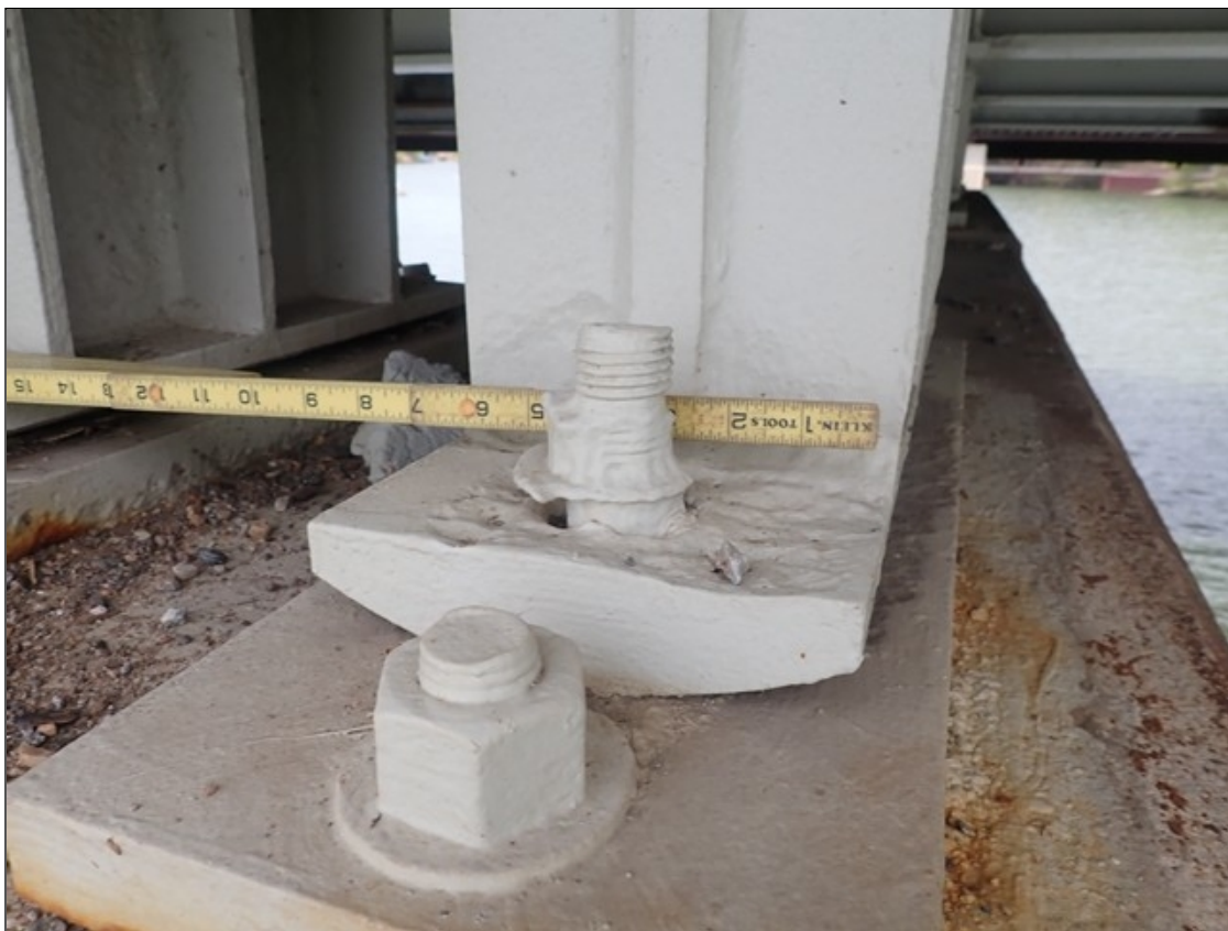
Span 6 Beam 2 Near Bearing - Protective System: PAINT FAILURE WITH ACTIVE CORROSION AND SECTION LOSS (CLEANED AND PAINTED)
