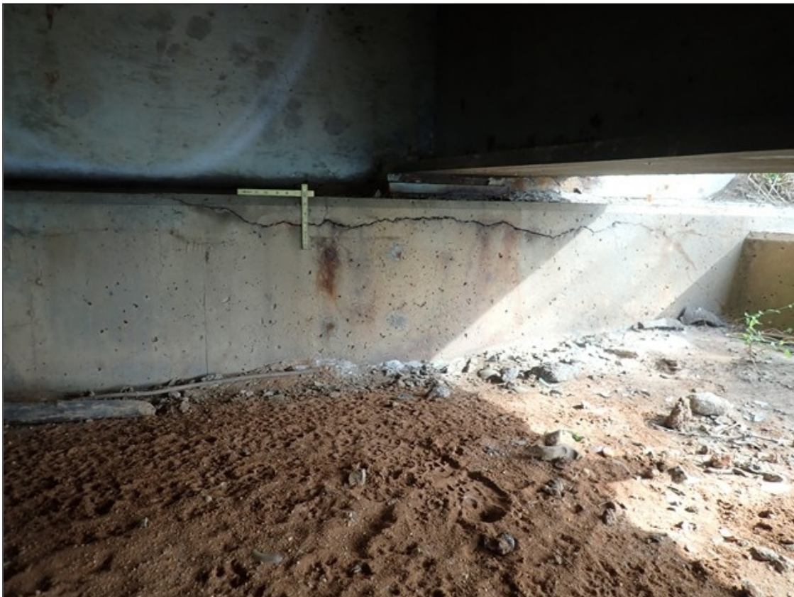
End Bent 1 Cap 1: ALONG LENGTH OF CAP BELOW BAY 1, HORIZONTAL CRACK [UP TO 10 FEET LONG X UP TO 1/8 INCHES] WITH 48 INCHES LONG X 8 INCHES HIGH AREA OF DELAMINATION
