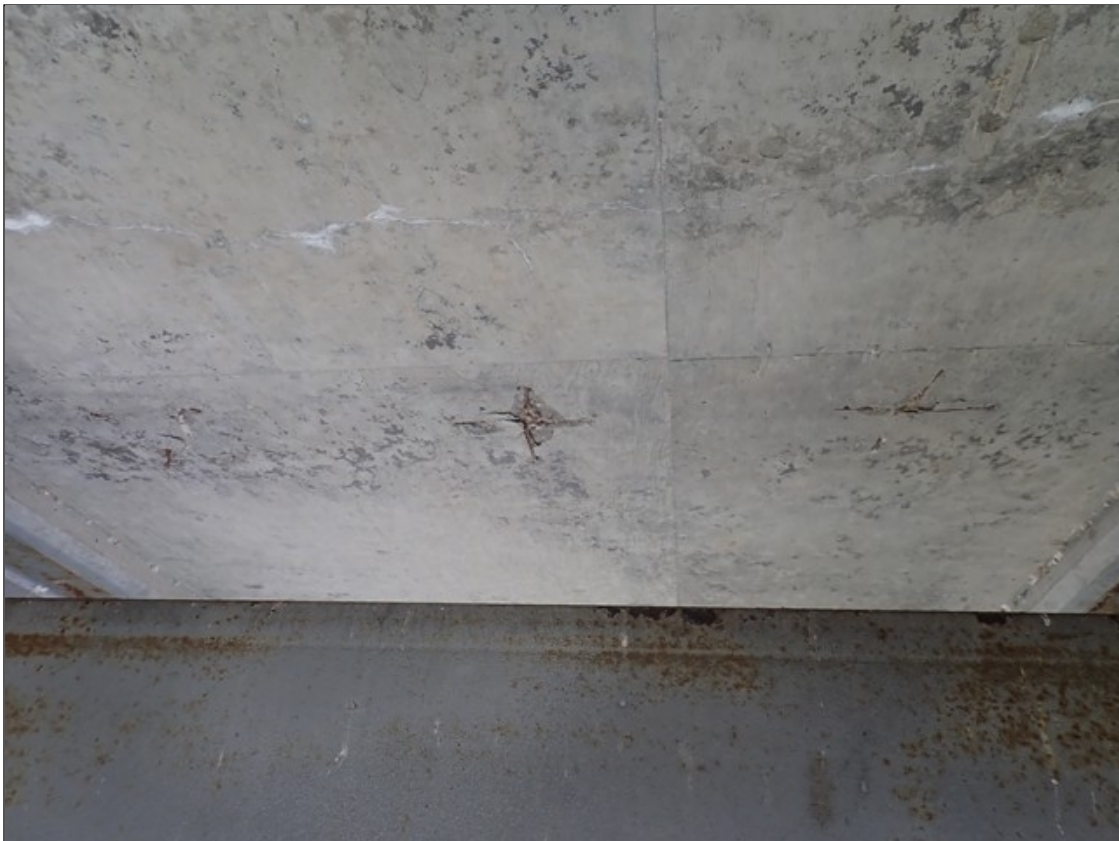
Span 8 Deck: (3) UP TO 9 INCH LONG X 9 INCH WIDE X 1/2 INCH DEEP SPALLS WITH EXPOSED REBAR ON BOTTOM OF DECK NEAR MIDSPAN (EACH BAY SIMILAR)
