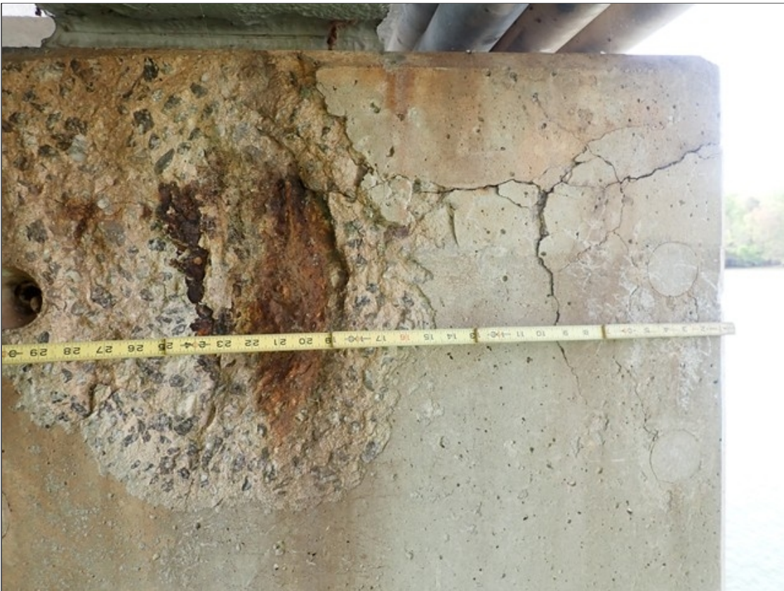
Bent 9 Cap 1: NORTH FACE AT WEST END, SPALL WITH EXPOSED REBAR AND AREA OF DELAMINATION [32 INCHES LONG X 20 INCHES HIGH X 1- 3/4 INCHES DEEP] WITH TWO [2] EXPOSED VERTICAL REBAR
