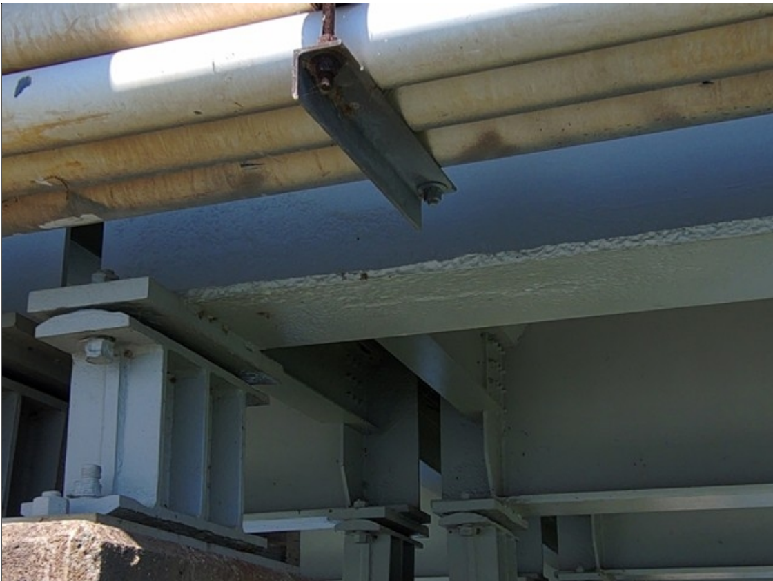
Span 2 Beam 1: SPAN 5 AT FAR END, CORROSION WITH SECTION LOSS; BOTTOM FLANGE: [6 FEET LONG X FULL WIDTH - 3/4 INCHES AVERAGE REMAINING] (CLEANED AND PAINTED) (PAR)
