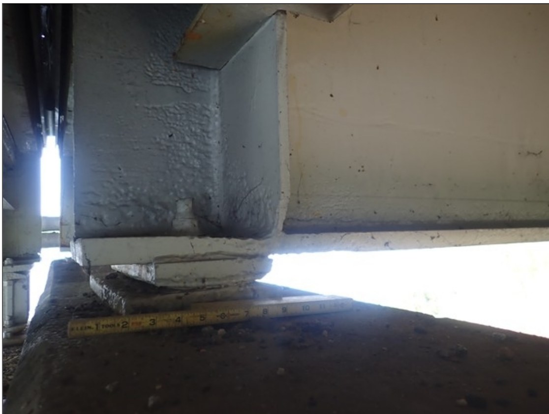
BENT 9 STEEL EXPANSION BEARING
