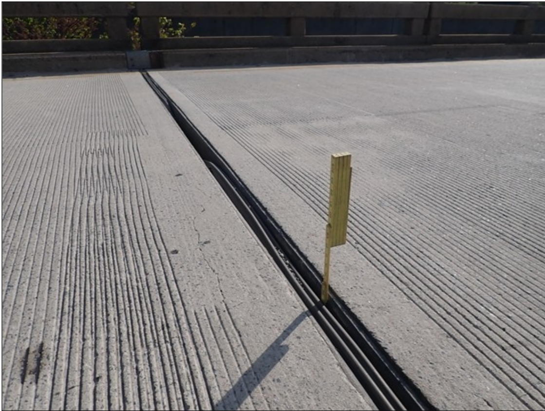
Span 10 Expansion Joint Bent 9: ALONG LENGTH OF JOINT, SEAL ADHESION FAILURE [ADHESION GREATER THAN 50%]
