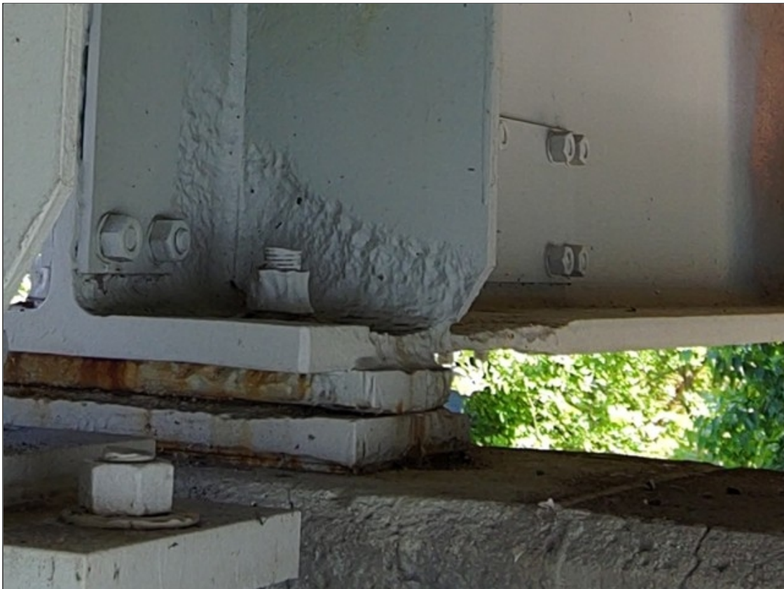
Span 1 Beam 4: 7/16 INCHES REMAINING X 8 INCHES WIDE ON BOTTOM LEFT FLANGE FOR 18 INCHES LONG AT BENT 1 (CLEANED AND PAINTED) (PAR)
