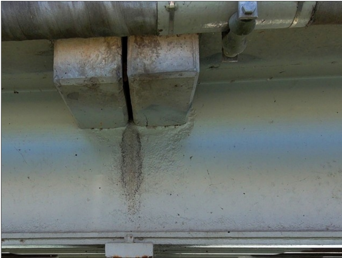
Span 2 Beam 4: OVER BENT 2, CORROSION WITH SECTION LOSS WEB OVER BEARING: [24 INCHES LONG X 17 INCHES HIGH - 5/8 INCHES AVERAGE REMAINING]; LOWER WEB: [7 FEET LONG X UP TO 5 INCHES WIDE - 5/8 INCHES AVERAGE REMAINING]; BOTTOM FLANGE: [11 FEET LONG X FULL WIDTH - 1 INCHES REMAINING] (CLEANED AND PAINTED) (PAR)
