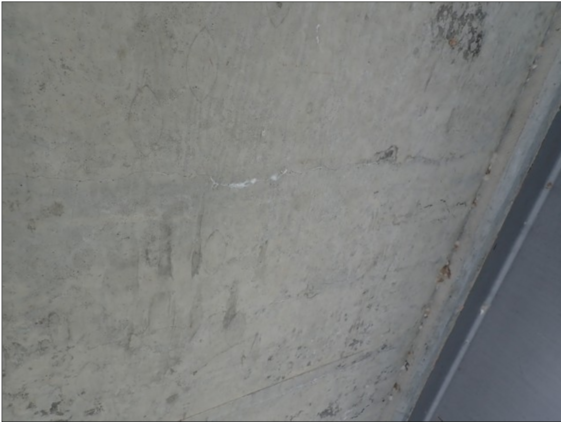
Span 8 Deck: HAIRLINE LONGITUDINAL AND TRANSVERSE CRACKS WITH EFFLORESCENCE ON BOTTOM OF DECK AT RANDOM THROUGHOUT EACH BAY
