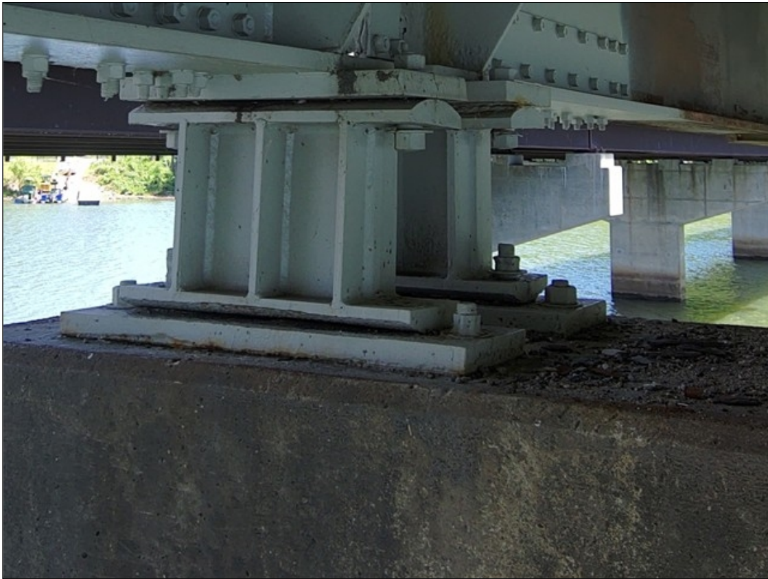
Span 6 Beam 4 - Beam 4 Near Bearing: WEST ROCKER BOLT IS MISSING (PAR)
