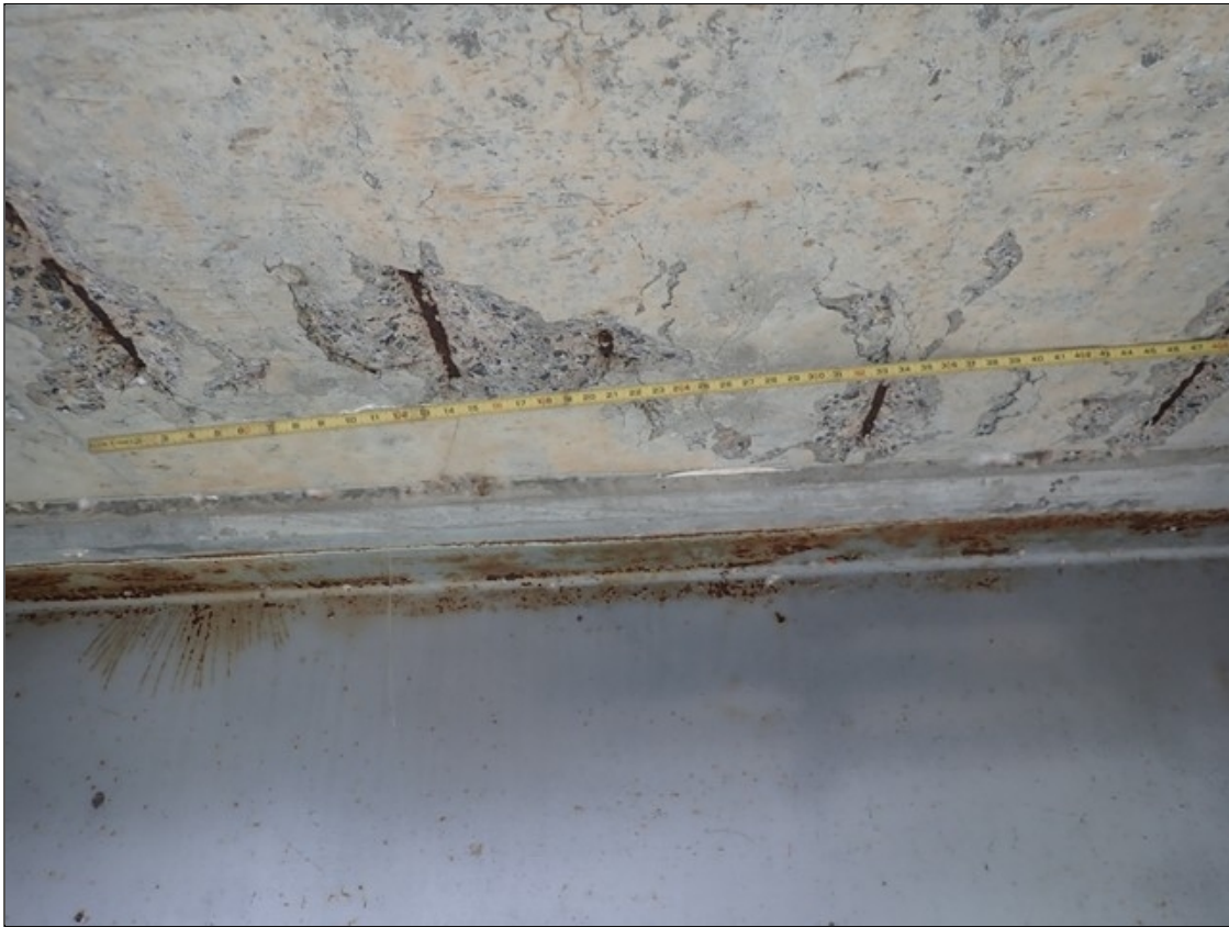
Span 8 Deck: 70 INCHES LONG X 24 INCHES WIDE X 1 INCH DEEP SPALLING WITH EXPOSED REBAR WITH NO SECTION LOSS AND DELAMINATION IN BAY 2 STARTING 10 FEET FROM BENT 8
