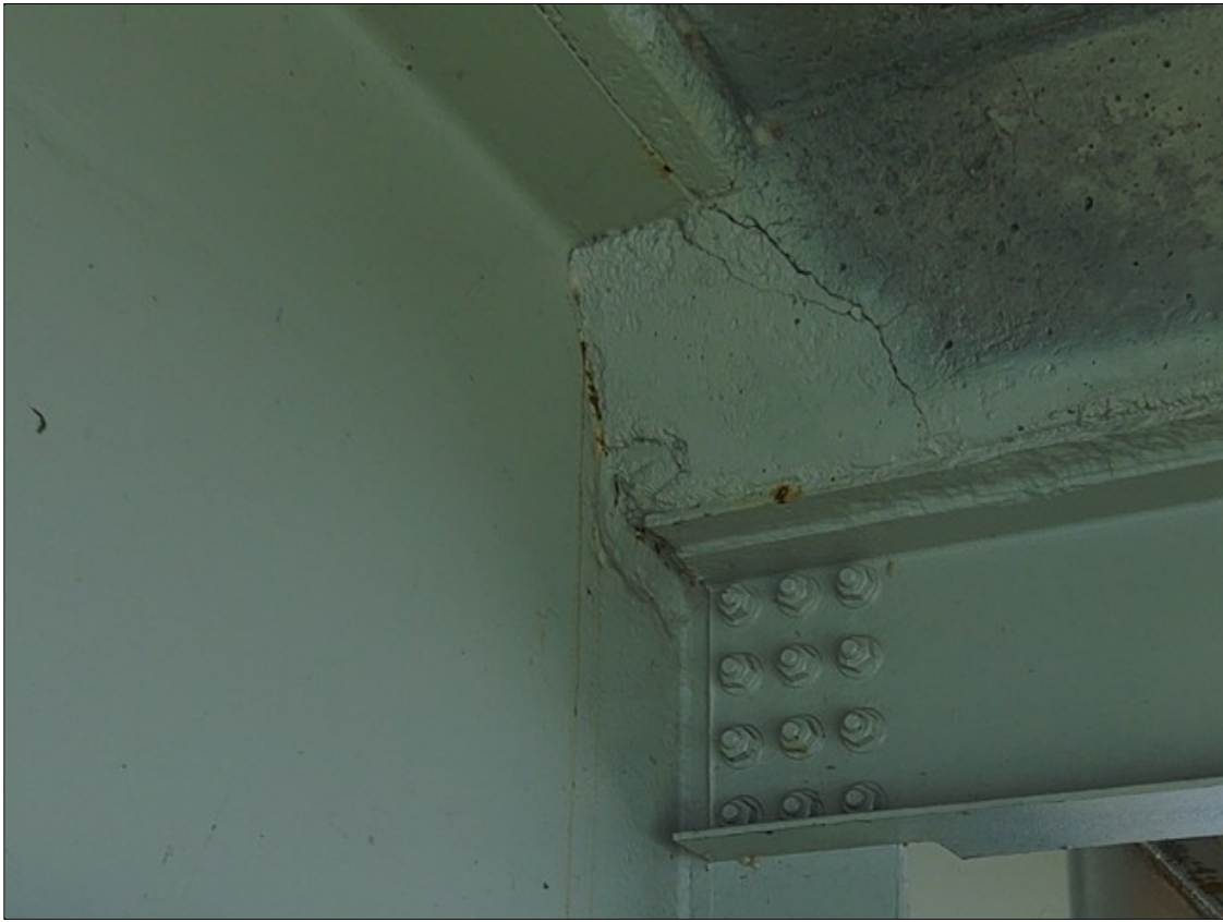
Span 6 Beam 4: UPPER WEB AT DIAPHRAGM AT BENT 6, CORROSION WITH SECTION LOSS [30 INCHES LONG X UP TO 12 INCHES HIGH - AVERAGE REMAINING 1/4 INCHES]; LOWER WEB [10 FEET LONG X UP TO 7 INCHES HIGH - AVERAGE REMAINING 3/8 INCHES] (CLEANED AND PAINTED) (PAR)
