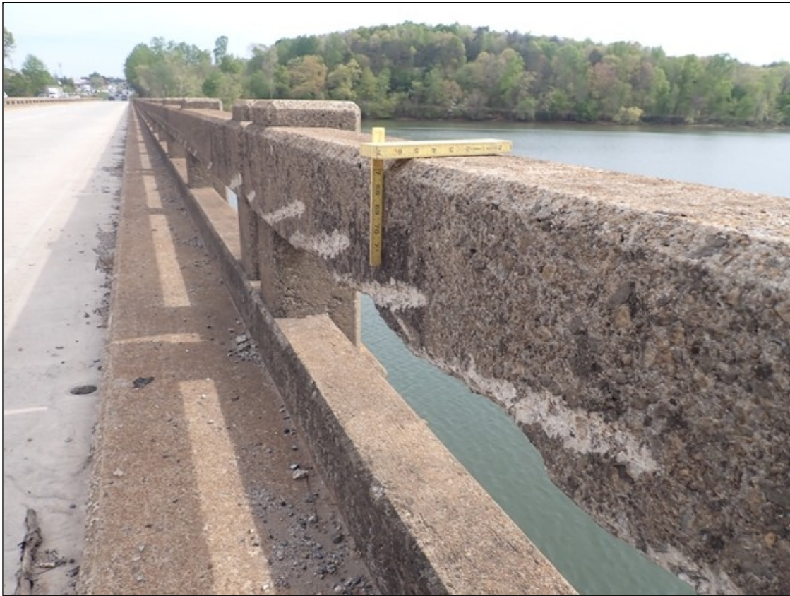
Span 9 Left Bridge Rail: 55 FEET AREA OF UP TO 15 INCH LONG X 3 INCH HIGH X 1 1/2 INCH DEEP SPALLS ON FAIL NEAR BENT 9
