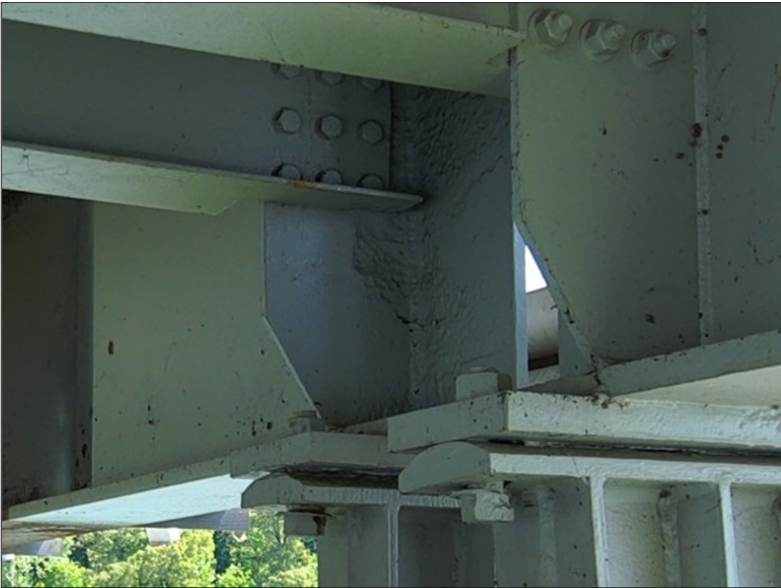
Span 2 Beam 1: 5 INCH LONG X 21 INCH HIGH AREA OF 1/8 INCH SECTION LOSS (3/8 INCH REMAINING) WITH NO RUST ON RIGHT STIFFENER AT BENT 5 (CLEANED AND PAINTED) (PAR)
