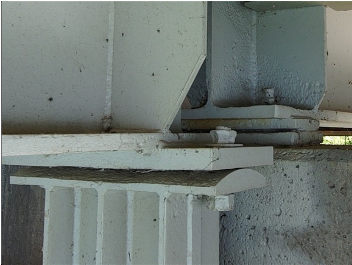
Span 2 Beam 2: SPAN 2 OVER BENT 1, CORROSION WITH SECTION LOSS: BOTH SIDES WEB OVER BEARING [8 INCHES LONG X 12 INCHES HIGH - AVERAGE REMAINING 5/8 INCHES]; LOWER WEB [2 FEET LONG X 1 FOOT HIGH- NO LOSS NOTED]; BOTTOM FLANGE [16 INCHES LONG X FULL WIDTH - NO LOSS NOTED] (CLEANED AND PAINTED) (PAR)
