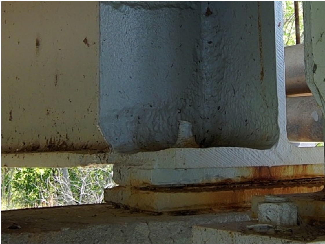
Span 1 Beam 1: 9 INCH LONG X 13 INCH HIGH AREA OF 1/8 INCH SECTION LOSS (3/8 INCH REMAINING) ON RIGHT SIDE OF STIFFENER AT BENT 1 (CLEANED AND PAINTED) (PAR)
