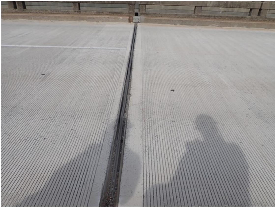
Span 2 Expansion Joint Bent 1: FULL LENGTH DIRT AND DEBRIS
