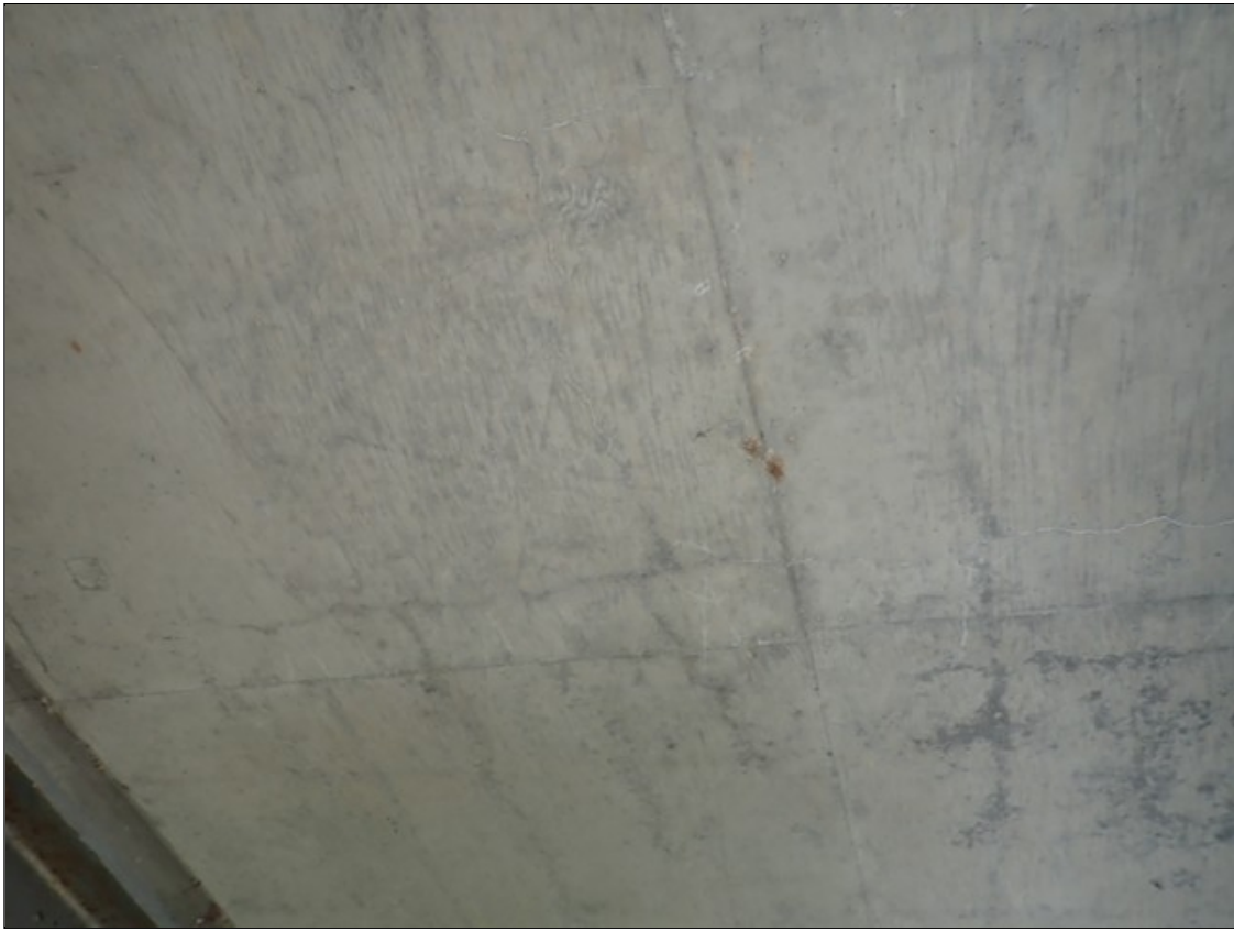
Span 9 Deck: HAIRLINE TRANSVERSE CRACKS ON BOTTOM OF DECK AT RANDOM THROUGHOUT IN BAYS 1 AND 3
