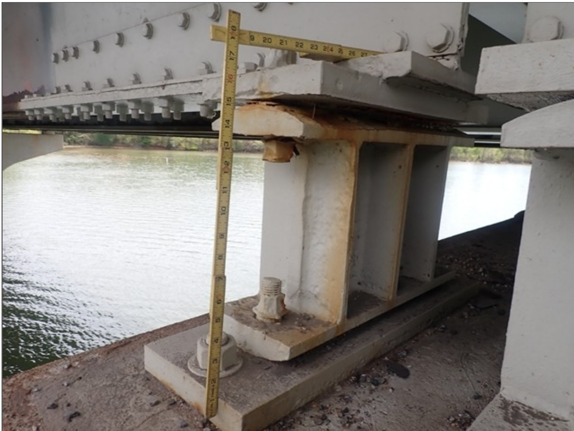
Span 2 Beam 4 Far Bearing - Protective System: PAINT FAILURE WITH ACTIVE CORROSION AND SECTION LOSS (CLEANED AND PAINTED)
