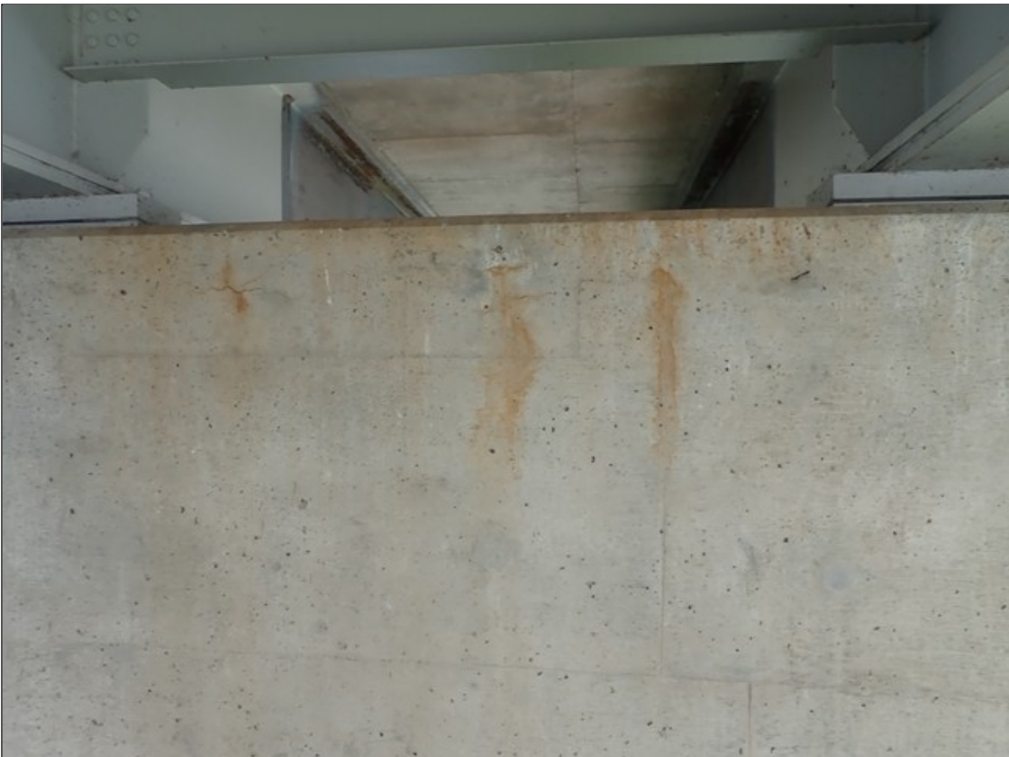
Bent 2 Cap 1: (3) UP TO 1 FEET LONG X 1 FEET WIDE AREA OF HAIRLINE HORIZONTAL AND VERTICAL CRACKS WITH EFFLORESCENCE AND RUST STAINS ON SPAN 3 FACE UNDER BAY 2
