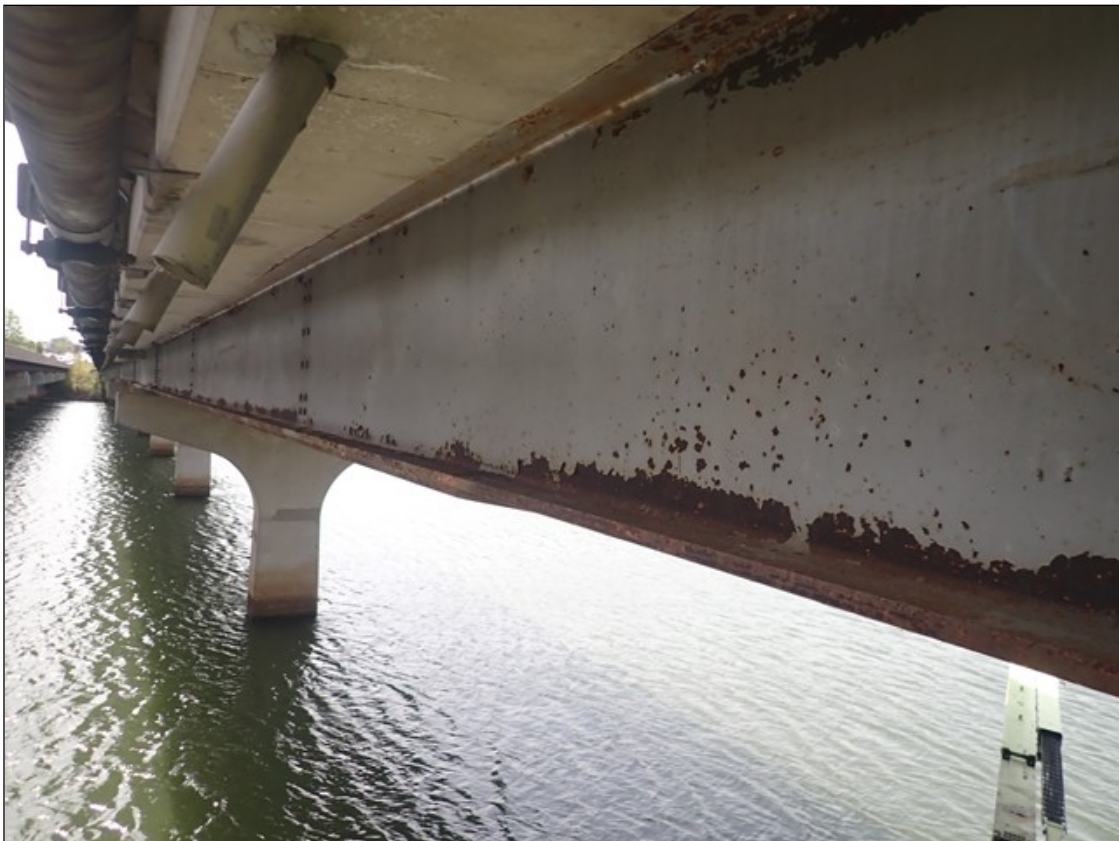
Span 6 Beam 4: PEELING PAINT WITH RUST AND SURFACE RUST ON BOTH FLANGES AND WEB AT RANDOM THROUGHOUT IN SPANS 6-9
