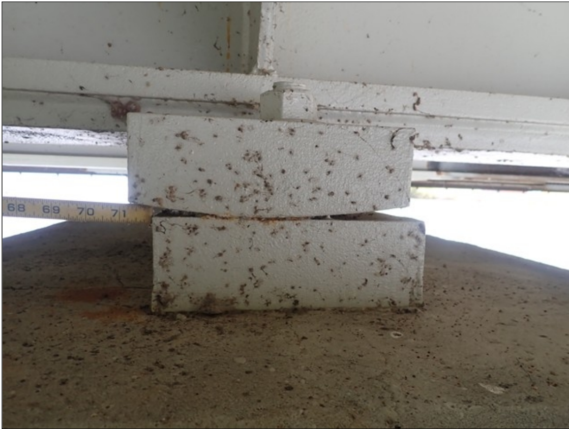
Span 6 Beam 2 Intermediate Bearing Bent 6: BEARING IS IN CONTRACTION [3/4 INCHES]
