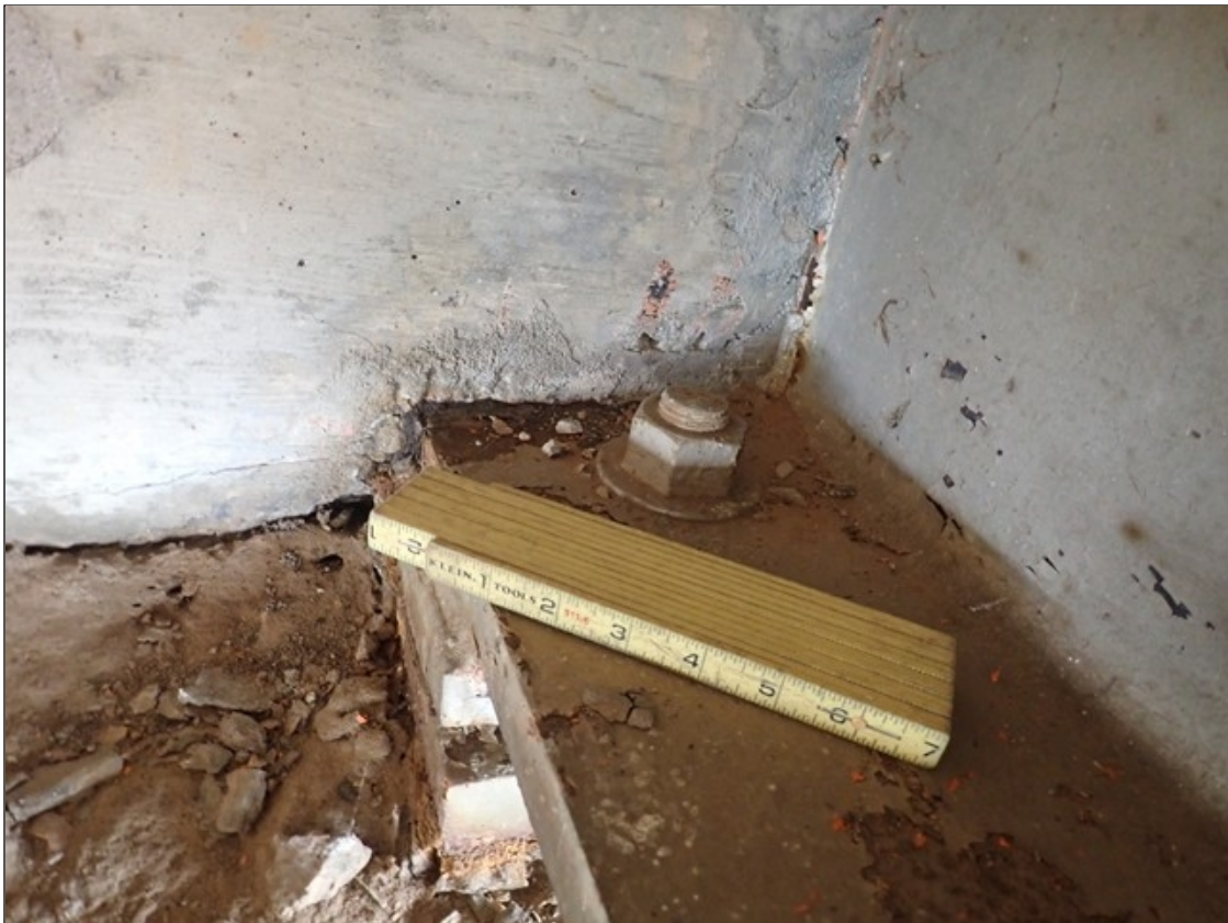
Span 1 Beam 1: 1 1/2 INCH LONG X 5 INCH HIGH AREA OF 1/8 INCH SECTION LOSS (1 1/8 INCH REMAINING) WITH NO RUST ON RIGHT SIDE OF BOTTOM FLANGE AT END BENT 1
