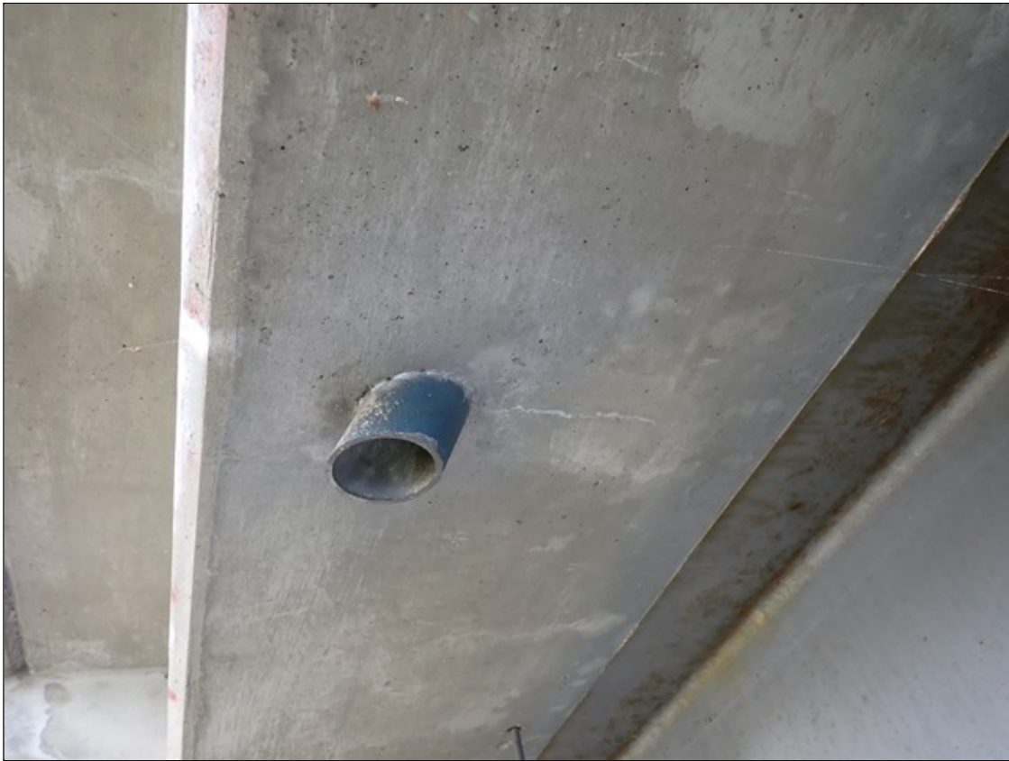
Span 10 Deck: ALONG LENGTH OF UNDERSIDE OF BOTH OVERHANGS AT DRAIN PIPES, MULTIPLE TRANSVERSE CRACKS [UP TO 3 FEET LONG X HAIRLINE]
