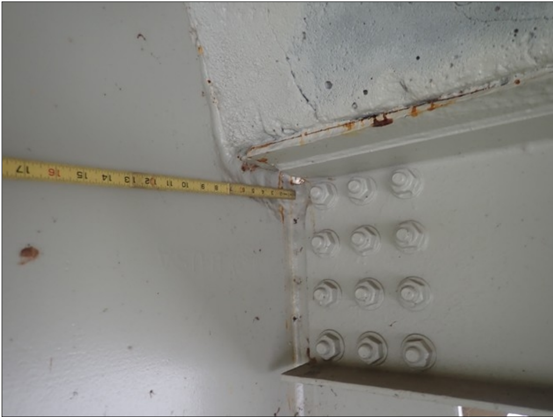
UPPER WEB AT BOTH FACES OF BENT 6 DECK HAUNCH, CORROSION WITH SECTION LOSS [18 INCHES LONG X UP TO 10 INCHES HIGH - AVERAGE REMAINING 1/4 INCHES]; LOWER WEB [20 INCHES LONG X 2 INCHES HIGH - SECTION LESS LESS THAN 1/16 INCHES] (CLEANED AND PAINTED) (PAR)
