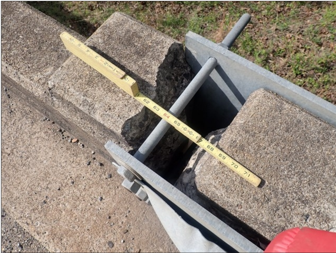
Span 10 Left Bridge Rail: (2) UP TO 10 1/2 INCHES LONG X 15 INCHES WIDE X 4 INCHES DEEP SPALL ON POST 12
