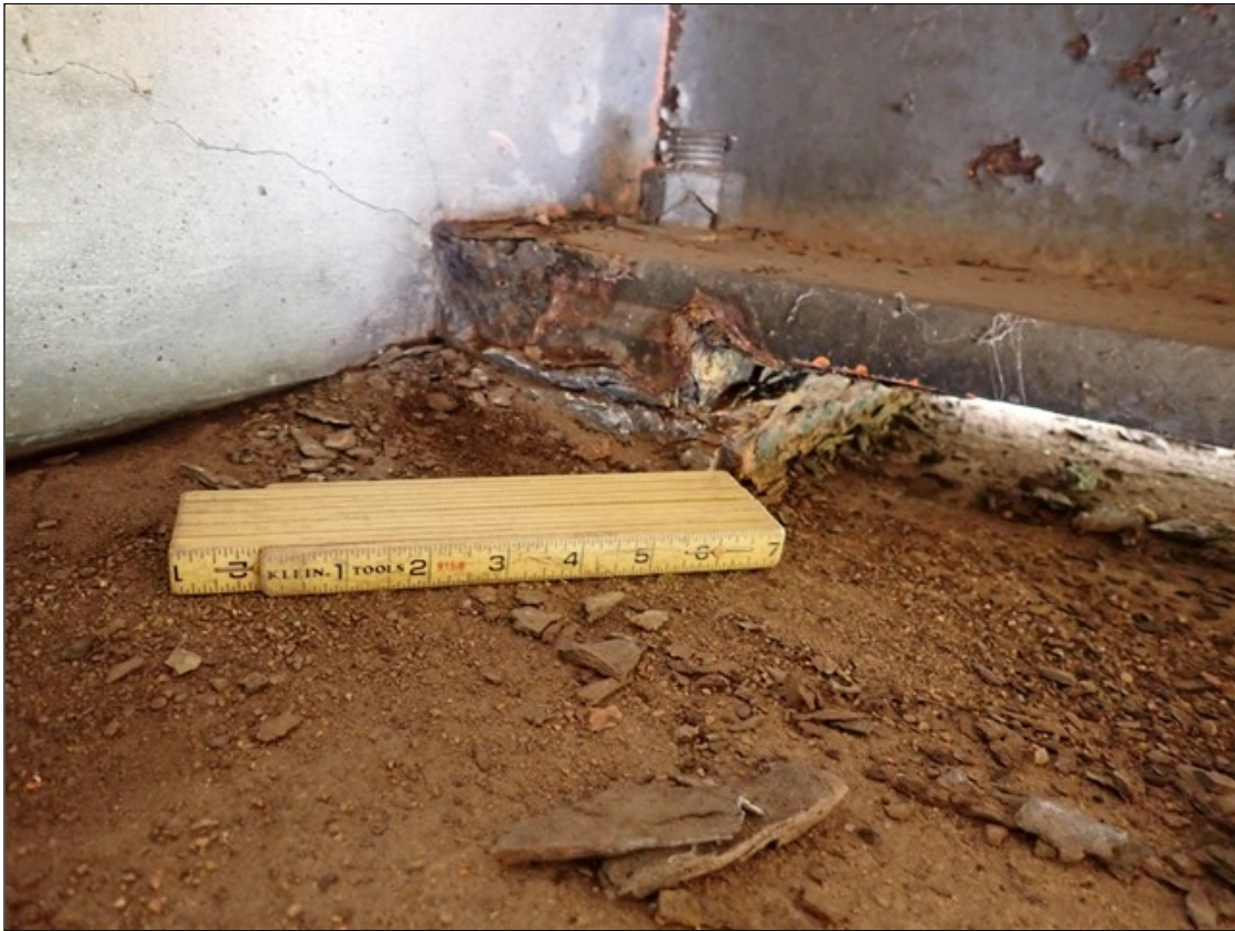
Span 10 Beam 4 - Beam 4 Far Bearing: PEELING PAINT WITH RUST
