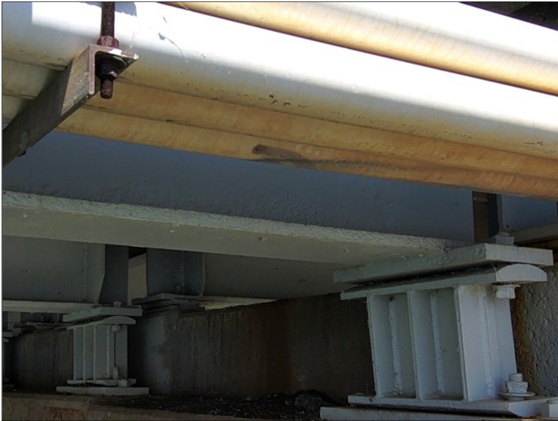
Span 2 Beam 1: SPAN 2 AT NEAR END, CORROSION WITH SECTION LOSS: LOWER WEB: [4 FEET LONG X 5 INCHES HIGH - 5/8 INCHES AVERAGE REMAINING]; BOTTOM FLANGE: [4 FEET LONG X FULL WIDTH - 1 INCHES AVERAGE REMAINING] (UPPER WEB REPAIRED IN 2022) (PAR)
