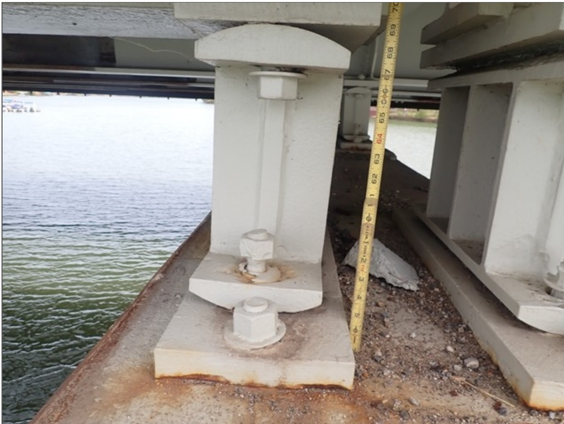
Span 6 Beam 1 Near Bearing: 3/8 INCHES ROTATION TO THE SOUTH
