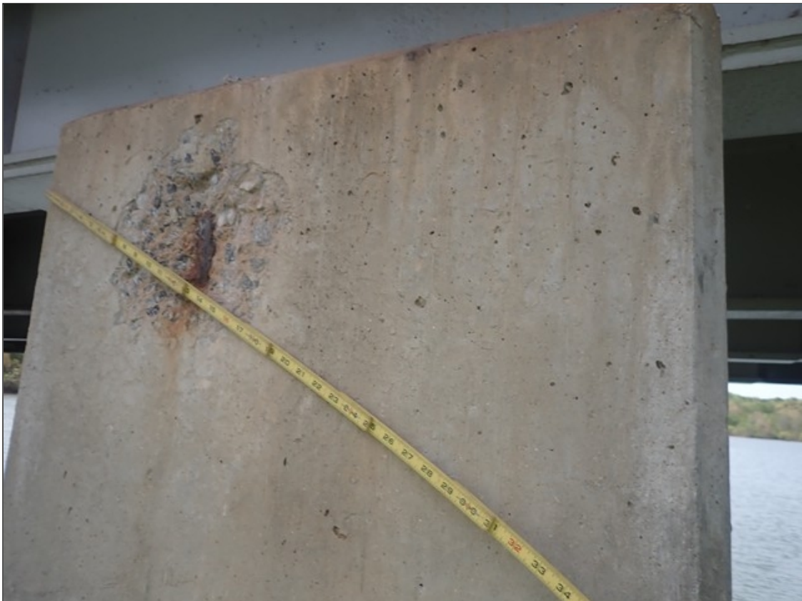
Bent 8 Cap 1: 12 INCHES LONG X 11 INCHES WIDE X 1 INCHES DEEP SPALL WITH EXPOSED REBAR ON EAST FACE (PAR)
