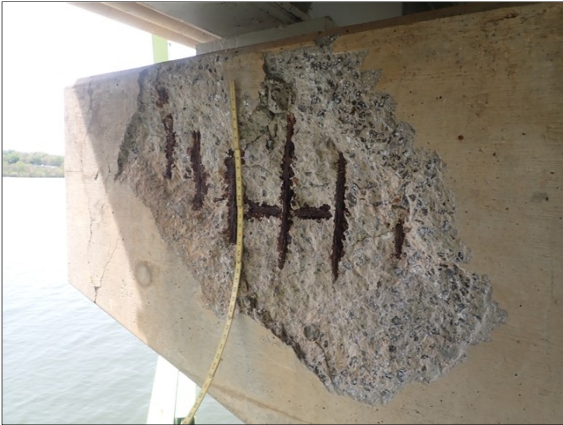
Bent 2 Cap 1: 42 INCHES WIDE X 33 INCHES TALL X 2 INCHES DEEP SPALLING WITH EXPOSED REBAR WITH SECTION LOSS WITH 14 INCH X 30 INCH AREA OF DELAMINATION ON SOUTH FACE UNDER GIRDER (PAR)
