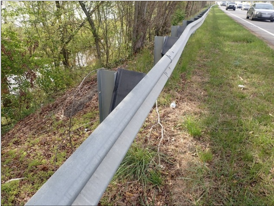
(2) AREAS OF 25 FEET OF IMPACT DAMAGE ON SOUTHWEST GUARDRAIL ACROSS FROM SOUTHEAST GUARDRAIL TERMINAL (PAR)
