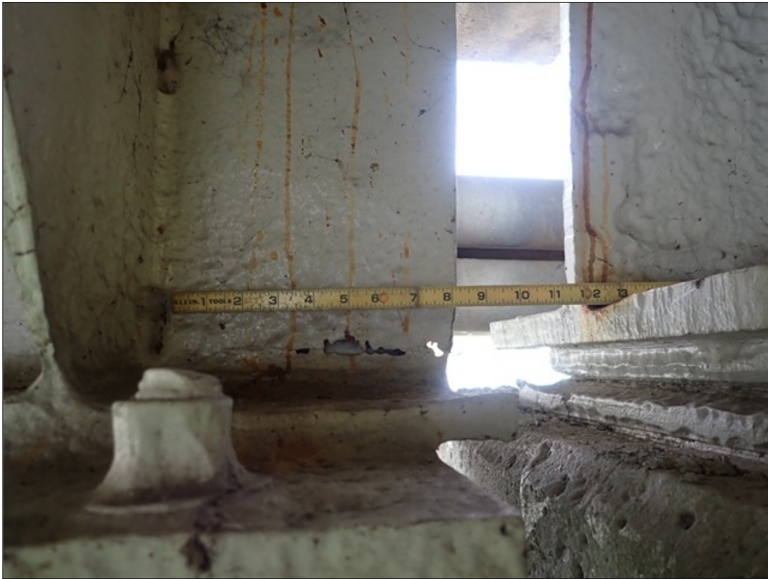
Span 6 Beam 1: 8 INCH LONG X 6 INCH HIGH AREA OF 3/16 INCH SECTION LOSS (5/16 INCH REMAINING) WITH NO RUST ON RIGHT STIFFENER IN SPAN 9 AT BENT 9 (CLEANED AND PAINTED) (PAR)
