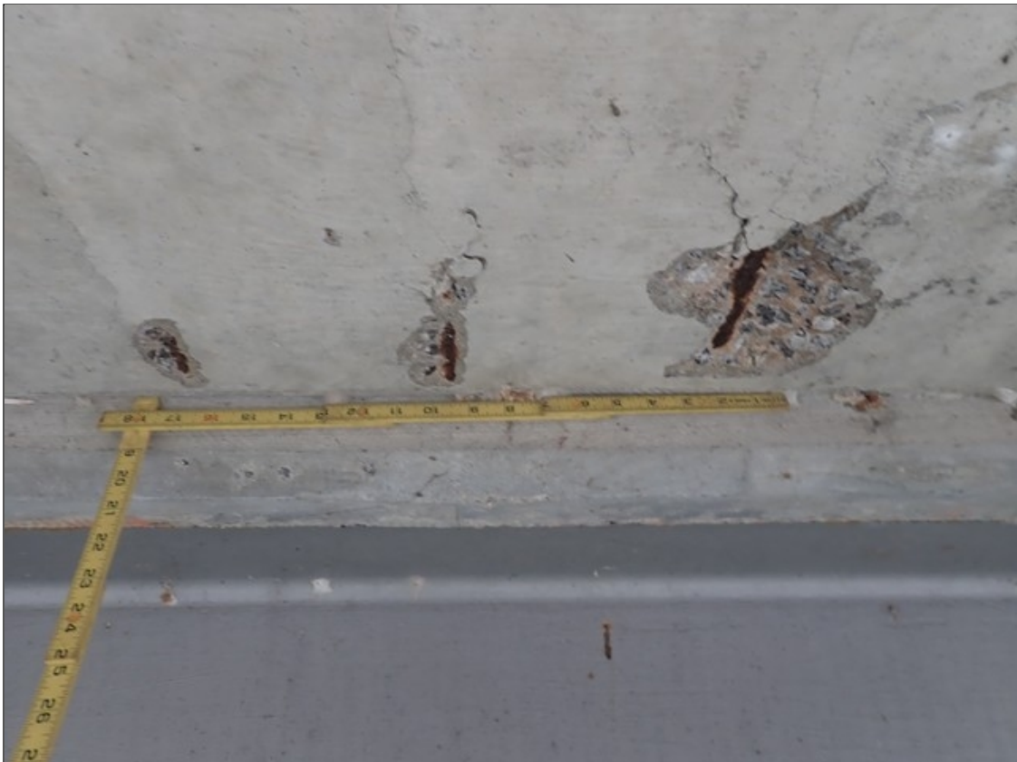
Span 8 Deck: (2) UP TO 6 INCH LONG X 2 INCH WIDE X 1/2 INCH DEEP SPALLS WITH EXPOSED REBAR ON BOTTOM OF DECK IN BAY 3, 30 FEET FROM BENT 8
