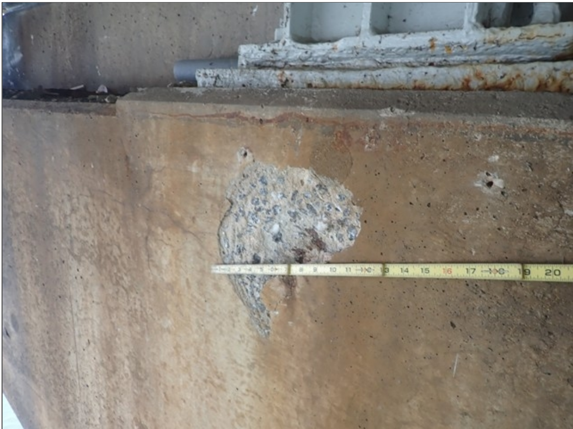
Bent 9 Cap 1: 12 INCH LONG X 12 INCH WIDE X 1/2 INCH DEEP SPALL AND AREA OF DELAMINATION ON SPAN 9 FACE UNDER BEAM 2
