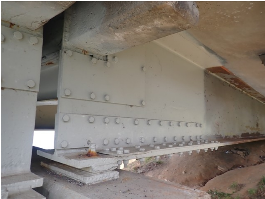
Span 10 Beam 4: MISSING BOLT ON WEB REPAIR PLATE AT BENT 9 (PAR)
