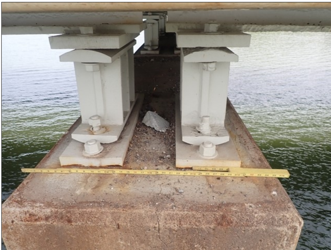
BENT 5 ROCKER BEARING
