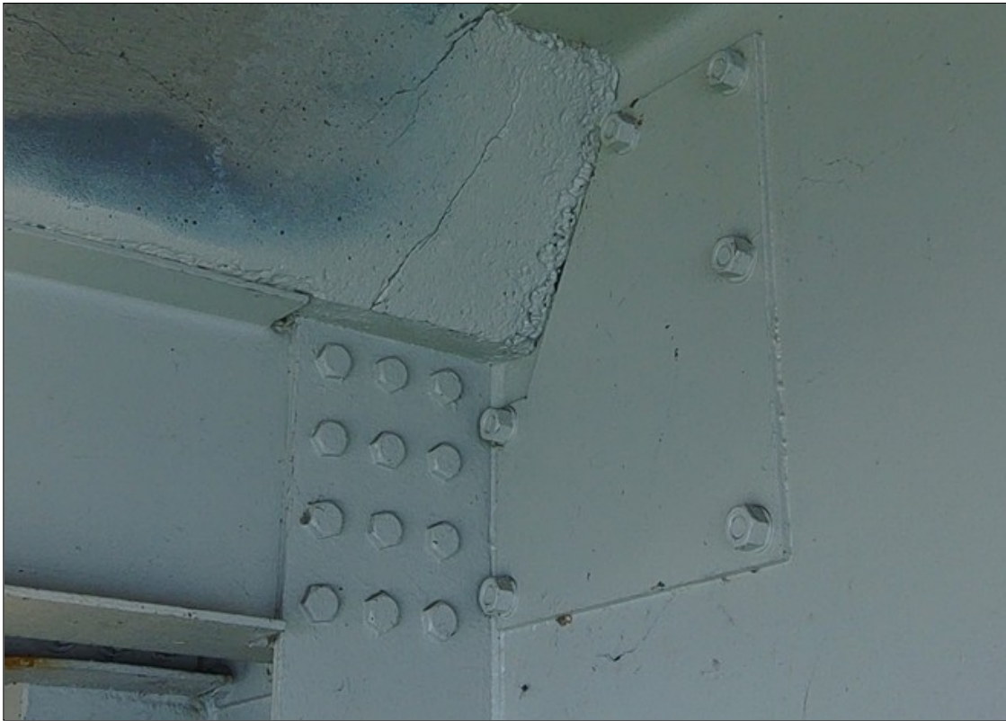
Span 6 Beam 4: IN SPAN 9 AT FAR END, ACTIVE CORROSION ABOVE PLATE, LEFT SIDE WEB AT DIAPHRAGM [12 INCHES LONG X 5 INCHES HIGH - AVERAGE REMAINING 1/2 INCHES] (CLEANED AND PAINTED) (PAR)
