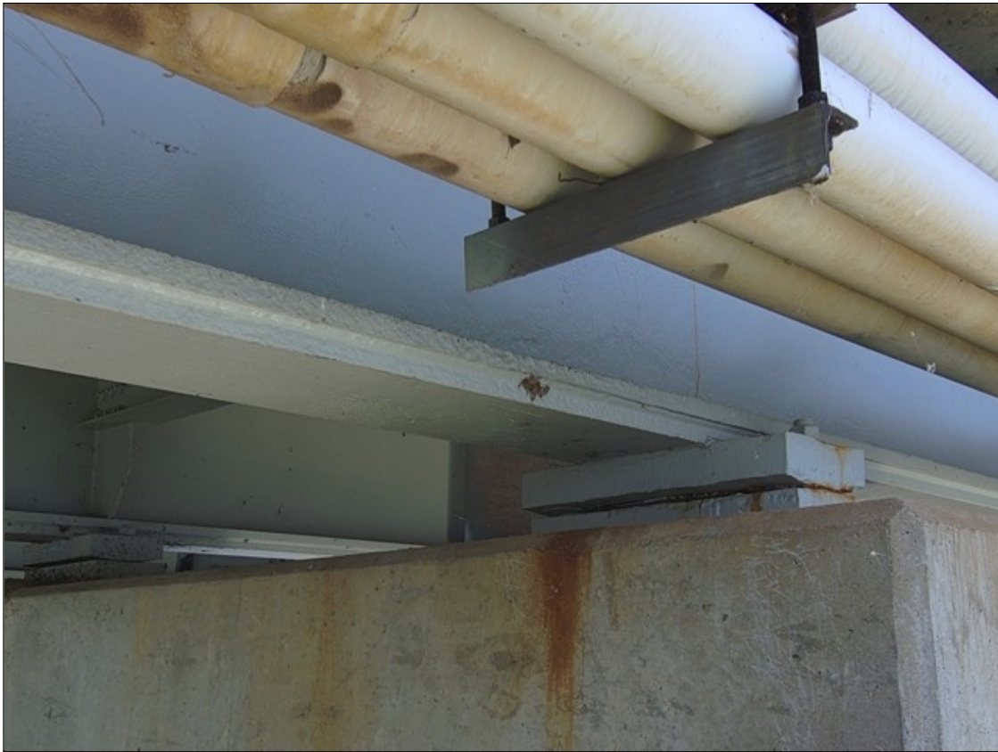
Span 6 Beam 1: AT BENT 6, CORROSION WITH SECTION LOSS, UPPER WEB AT DIAPHRAGM [18 INCHES LONG X 10 INCHES HIGH - AVERAGE REMAINING 1/4 INCHES]; LOWER WEB [6 FEET LONG X 4 INCHES WIDE - AVEERAGE REMAINING 5/16 INCHES]; BOTTOM FLANGE [2 FEET LONG X FULL WIDTH - 1 INCHES REMAINING] (CLEANED AND PAINTED WITH NO RUST) (PAR)
