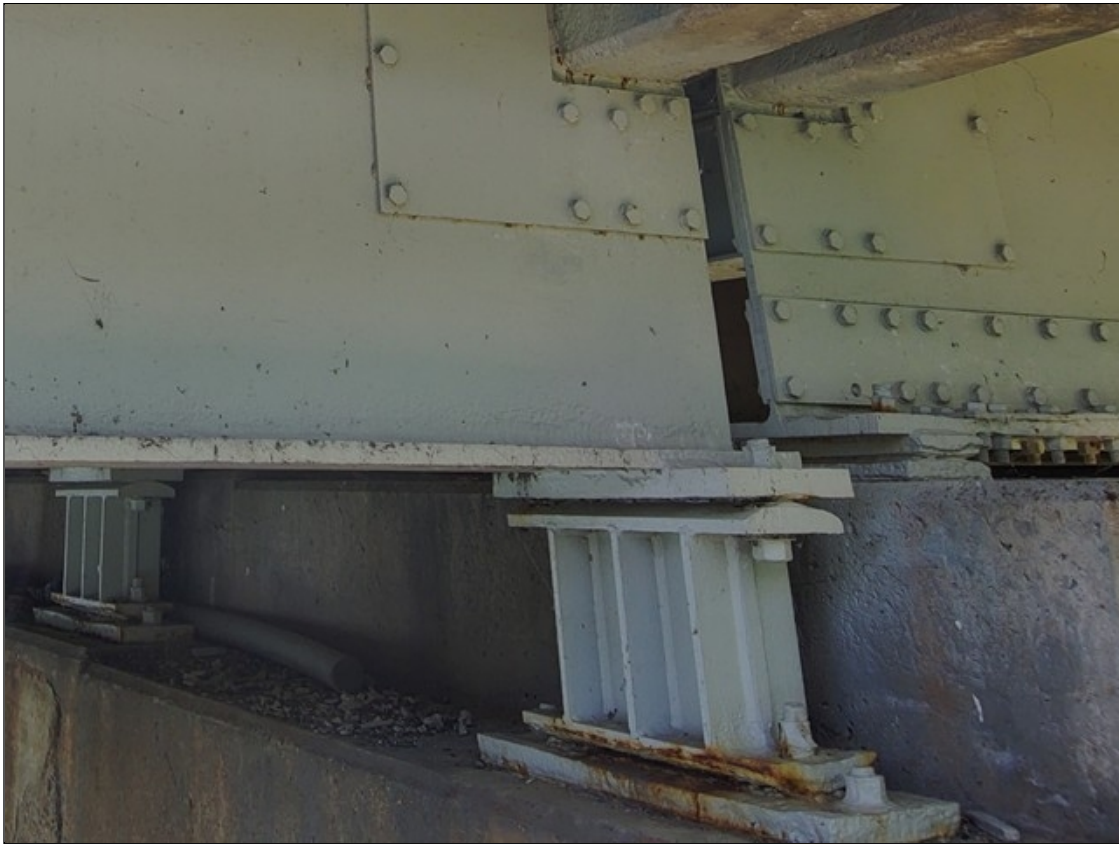
Span 6 Beam 4: IN SPAN 9 AT FAR END, CORROSION, LOWER WEB [34 INCHES LONG X 2 INCHES HIGH - AVERAGE REMAINING 11/16 INCHES]; BOTTOM FLANGE [32 INCHES LONG X UP TO 6 INCHES WIDE- AVERAGE REMAINING 7/8 INCHES] (PAINTED WITH NO RUST) (PAR)
