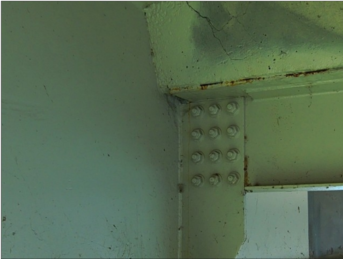
Span 2 Beam 1: AT BENT 2, CORROSION WITH SECTION LOSS UPPER WEB AT DIAPHRAGM: [18 INCHES LONG X 13 INCHES WEB - 3/8 INCHES AVERAGE REMAINING]; LOWER WEB: [3 FEET LONG X 4 INCHES WIDE - LOSS LESS THAN 1/16 INCHES]; BOTTOM FLANGE: [2 FEET LONG X FULL WIDTH - SECTION LOSS LESS THAN 1/16 INCHES] (PAR)
