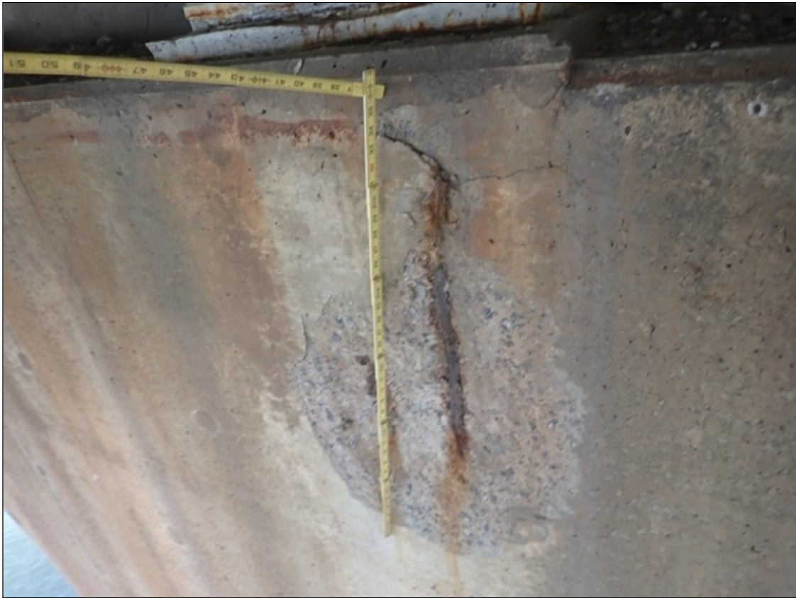
Bent 9 Cap 1: SOUTH FACE AT BEAM 3, SPALL WITH EXPOSED REBAR [22 INCHES WIDE X 34 INCHES TALL X UP TO 2 INCHES DEEP] WITH TWO [2] EXPOSED VERTICAL REBAR WITH SECTION LOSS (PAR)
