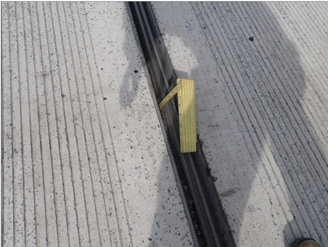
Span 6 Expansion Joint Bent 5: LOSS OF ADHESION OVER 80 PERCENT OF THE FULL LENGTH
