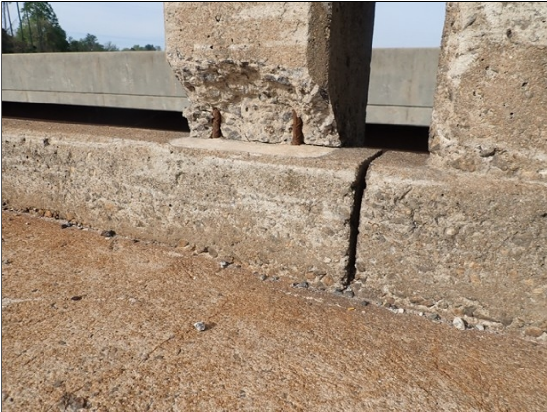
Span 7 Right Bridge Rail: 10 INCH X 4 INCH X 3 INCH DEEP SPALL WITH EXPOSED REBAR ON POST 4
