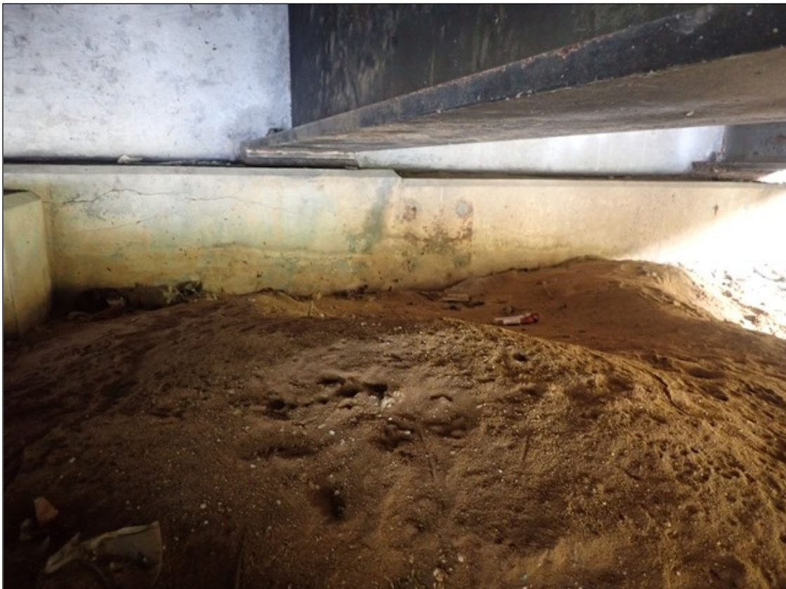
End Bent 2 Cap 1: 11 FEET LONG X UP TO 1/16 INCHES WIDE HORIZONTAL CRACKS UNDER BAYS 2 AND 3
