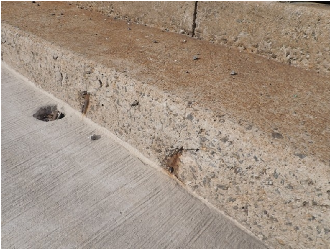
Span 3 Right Bridge Rail: 16 FEET FROM BENT 2, TWO [2] SPALLS [UP TO 6 INCHES LONG X 2 INCHES HIGH X 1/4 INCHES DEEP] WITH TWO [2] EXPOSED RUSTED REINFORCING [NO LOSS NOTED]
