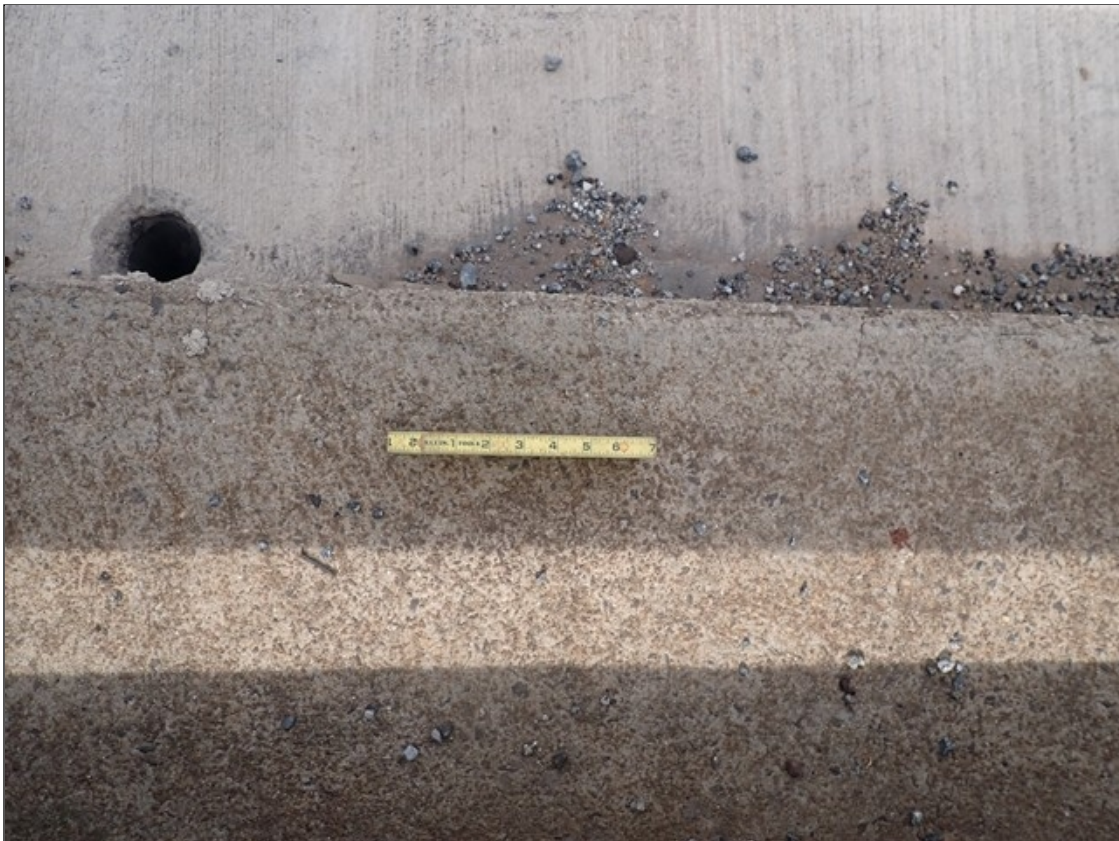
Span 9 Left Bridge Rail: HAIRLINE TRANSVERSE CRACKS ON RAIL AND CURB AT RANDOM THROUGHOUT
