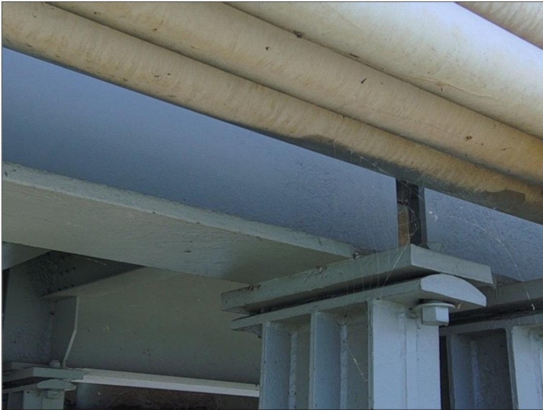
Span 6 Beam 1: 15 INCHES LONG X 10 INCHES HIGH AREA OF 1 INCHES SECTION LOSS (1/4 INCHES REMAINING) ON LEFT SIDE OF WEB IN SPAN 6 AT BENT 5 (CLEANED AND PAINTED) (PAR)
