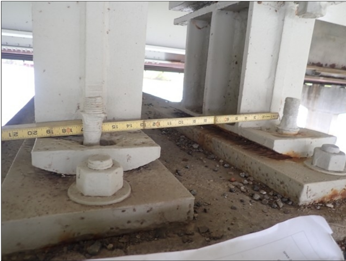
Span 2 Beam 2 Far Bearing: BEARING EXHIBITS PACK RUST [3/16 INCHES] AND CORROSION WITH SECTION LOSS [SECTION LOSS UP TO 1/16 INCHES] (CLEANED AND PAINTED)
