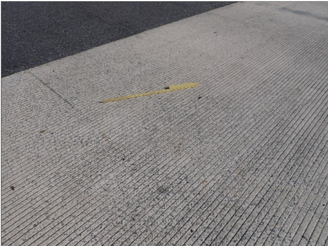
Span 10 Concrete Wearing Surface: 1/32 INCHES WIDE MAP CRACKING IN WEARING SURFACE PARTICULARLY AT JOINTS
