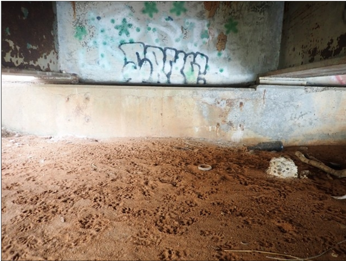
End Bent 1 Cap 1: 60 INCHES LONG X 9 INCHES HIGH X 1 INCHES DEEP SPALL AND AREA OF DELAMINATION WITH 7 FEET LONG UP TO 1/8 INCHES HORIZONTAL CRACK UNDER BAY 3
