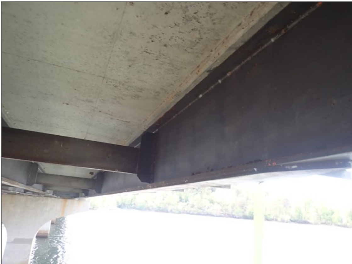
Span 6 Beam 1: PEELING PAINT WITH RUST AND SURFACE RUST ON BOTH FLANGES AND WEB AT RANDOM THROUGHOUT IN SPANS 6-9
