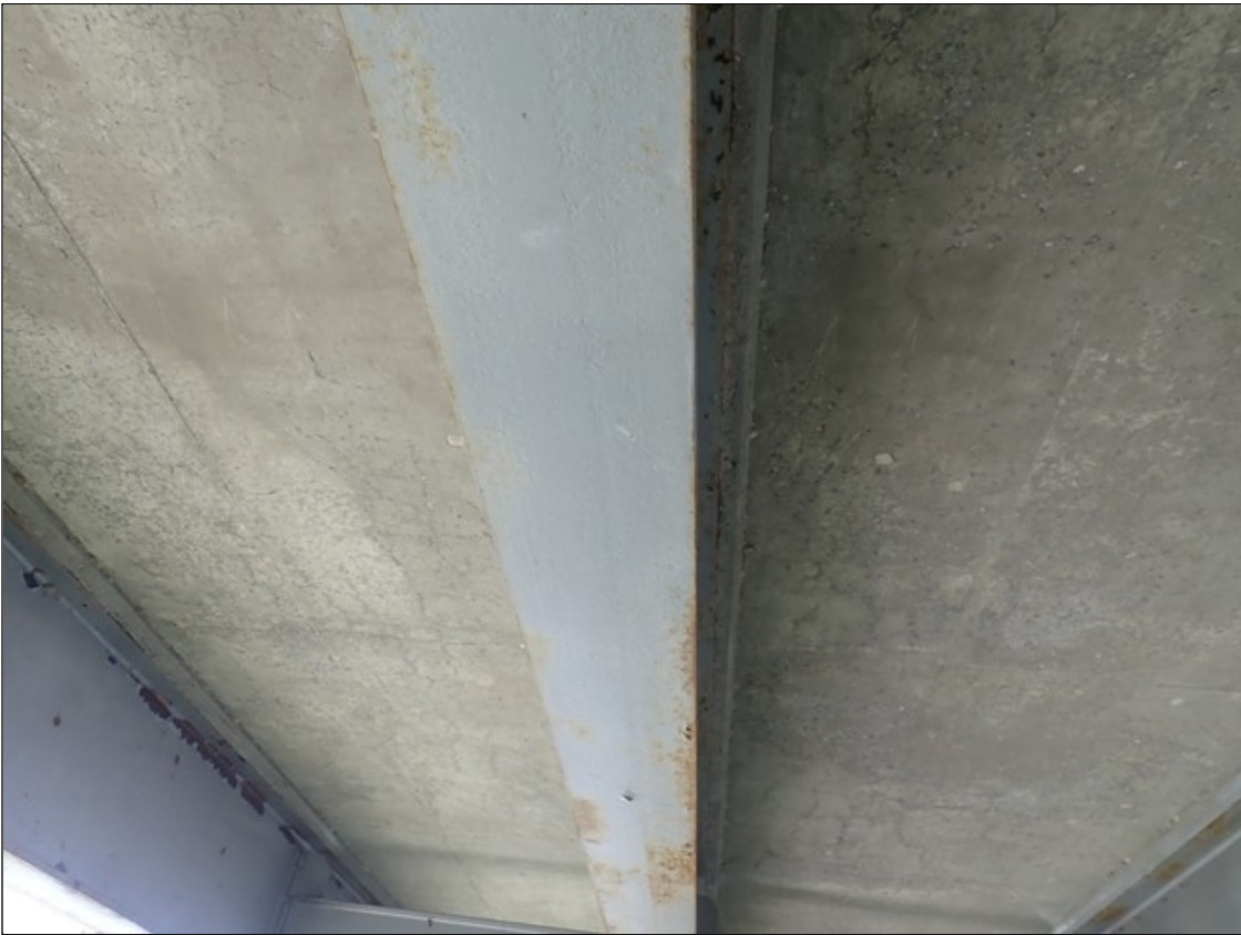
Span 4 Deck: WEATHERED CONCRETE WITH EXPOSED AGGREGATE WITH HAIRLINE MAP CRACKING ON BOTTOM OF DECK AT RANDOM THROUGHOUT
