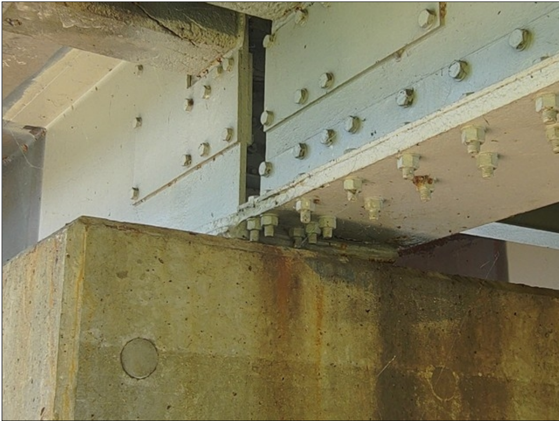
Span 10 Beam 4: AT NEAR END, CORROSION WITH SECTION LOSS, UPPER WEB AT DIAPHRAGM: [12 INCHES LONG X 1 INCHES WIDE - AVERAGE REMAINING 1/4 INCHES] ; LOWER WEB: [19 INCHES LONG X 3 INCHES HIGH - AVERAGE REMAINING 7/16 INCHES]; BOTTOM FLANGE: [20 INCHES LONG X 5 INCHES WIDE - AVERAGE REMAINING 7/8 INCHES] (REPAIRED IN 2022) (PAR)
