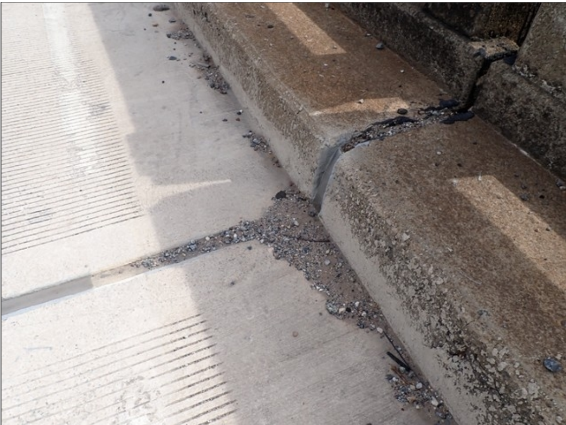
Span 8 Joint Bent 7: 2 FEET DIRT AND DEBRIS
