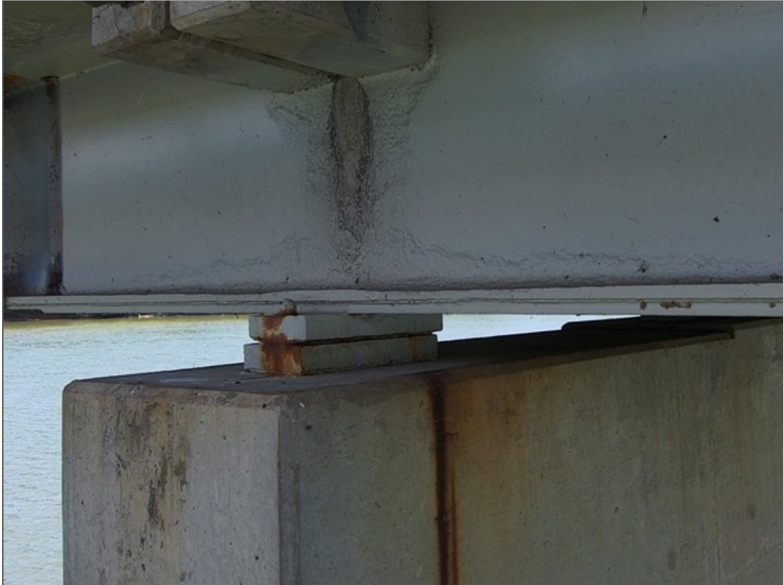
Span 6 Beam 4: 10 FEET LONG X 5 INCHES HIGH AREA OF UP TO 5/8 INCHES SECTION LOSS (7/8 INCHES REMAINING) ON RIGHT SIDE OF BOTTOM FLANGE IN SPAN 7 AT BENT 6 (CLEANED AND PAINTED) (PAR)
