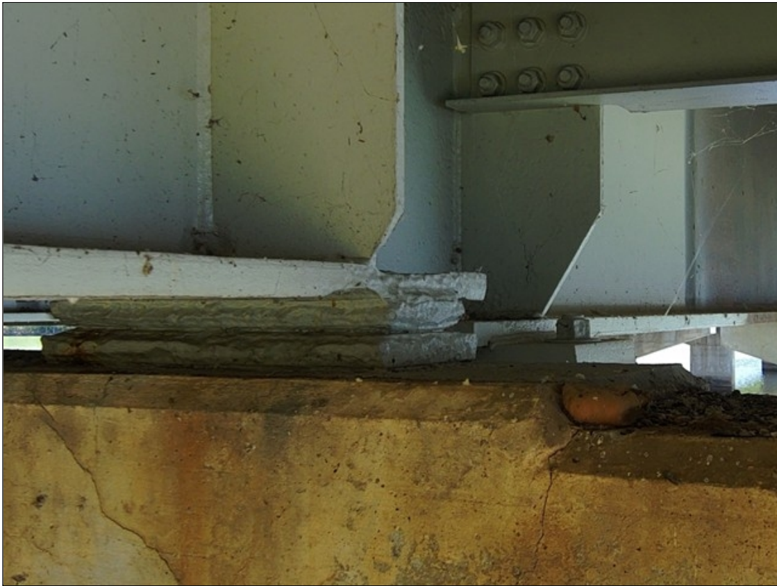
Span 10 Beam 2: 10 INCH LONG X 3 INCH HIGH AREA OF 1/8 INCH SECTION LOSS (3/8 INCH REMAINING) WITH NO RUST ON BOTH STIFFENERS AT BENT 9 (PAR) (CLEANED AND PAINTED)
