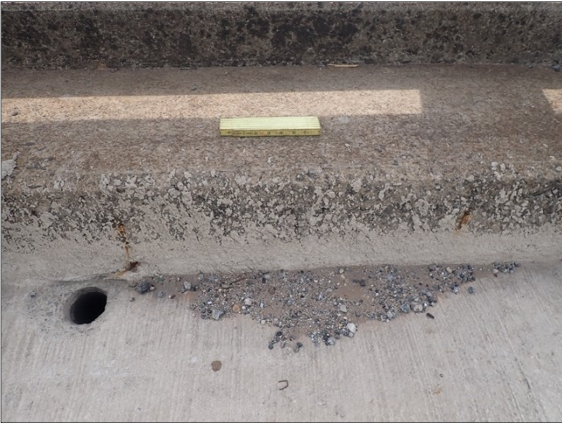
Span 8 Left Bridge Rail: ALONG LENGTH OF RAIL AND CURB, FIVE [5] SPALLS [UP TO 6 INCHES X 2 INCHES X 1/2 INCHES DEEP] EXPOSING FIVE [5] EXPOSED RUSTED REINFORCING [NO SECTION LOSS NOTED]
