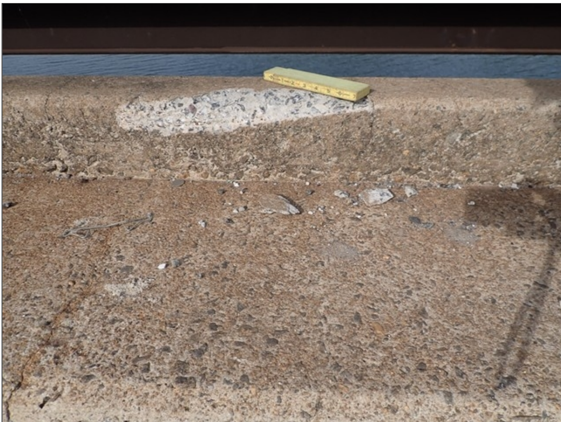
Span 3 Right Bridge Rail: 18 INCH LONG X 1 INCH HIGH X 2 INCH WIDE SPALL
