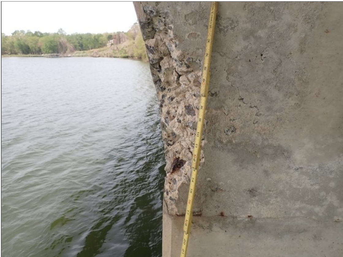
Bent 6 Pile 1: 5 INCHES WIDE X 4 INCHES LONG X 18 INCHES TALL SPALL WITH EXPOSED STEEL ON SOUTHWEST CORNER
