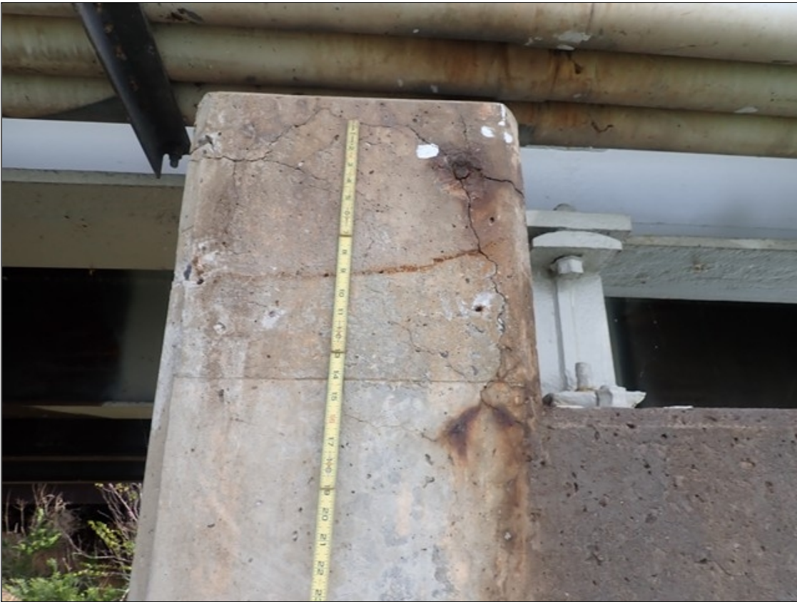
Bent 9 Cap 1: WEST FACE OF CAP, DELAMINATION/SPALL [18 INCHES LONG X 18 INCHES HIGH X UP TO 3/4 INCHES DEEP] WITH RUST STAIN
