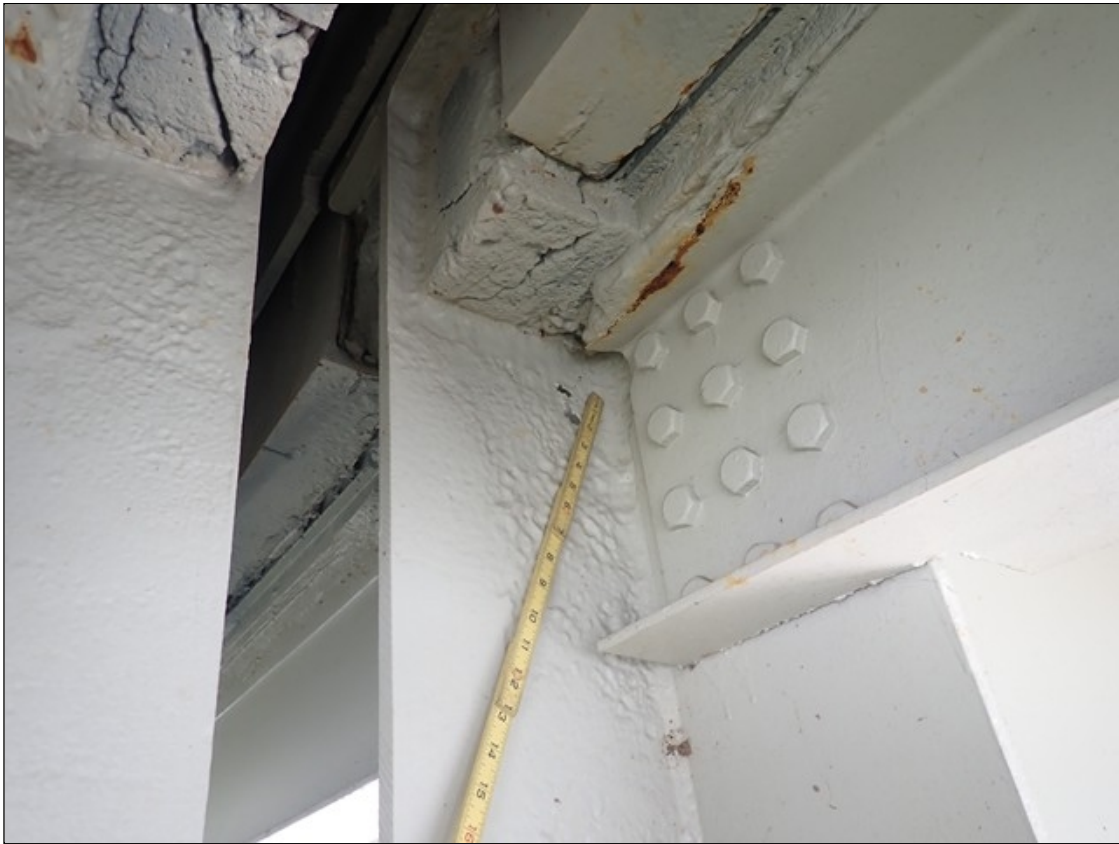
Span 2 Beam 2: 9 INCHES LONG X 24 INCHES HIGH AREA OF 3/16 INCHES SECTION LOSS (9/16 INCHES REMAINING) WITH 1 INCH LONG X 2 INCH HIGH AREA OF 100% SECTION LOSS ON WEB IN SPAN 5 AT BENT 5 (CLEANED AND PAINTED) (PAR)
