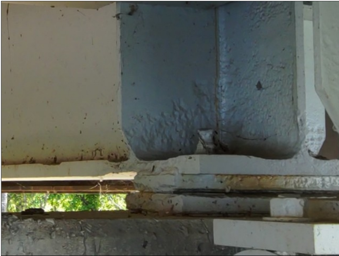
Span 1 Beam 2: 9 INCH LONG X 5 INCH HIGH AREA OF 1/8 INCH SECTION LOSS (3/8 INCH REMAINING) WITH NO RUST ON BOTH SIDES OF STIFFENER AT BENT 1 (PAR) (CLEANED AND PAINTED)
