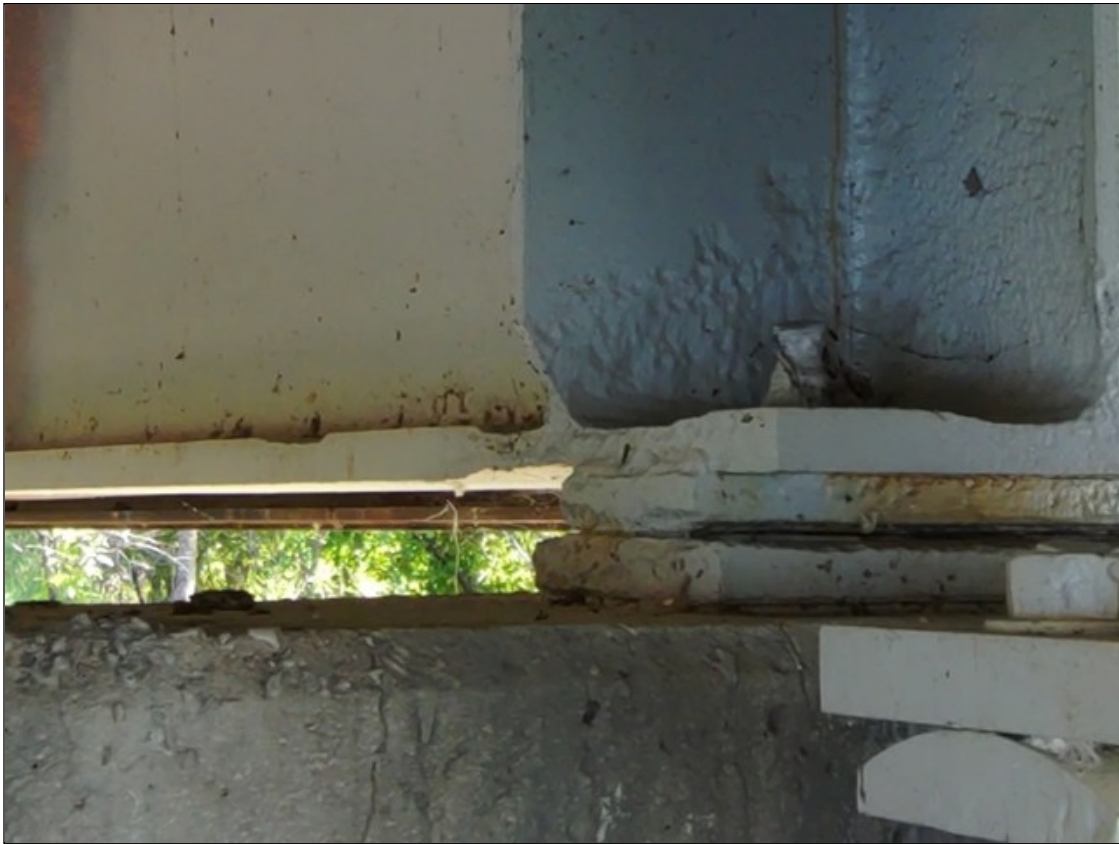
Span 1 Beam 2: AT FAR END, CORROSION WITH SECTION LOSS: BOTTOM RIGHT FLANGE [(2) UP TO 8 INCHES LONG X FULL WIDTH - AVERAGE REMAINING 3/4 INCHES], WEB OVER BEARING [9 INCHES LONG X FULL HEIGHT - AVERAGE REMAINING 1/2 INCHES] (CLEANED AND PAINTED) (PAR)
