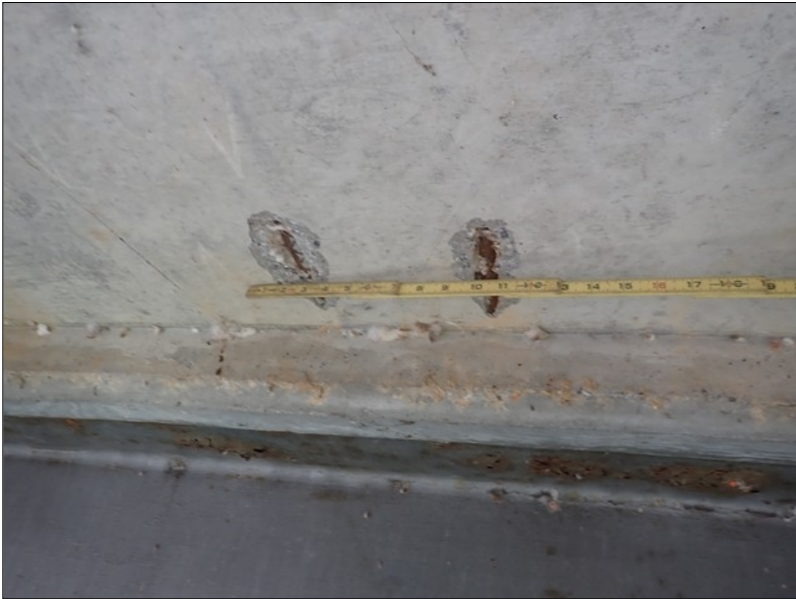
Span 9 Deck: (5) UP TO 7 INCHES LONG X 3 INCHES WIDE X 1/2 INCHES DEEP SPALLS WITH EXPOSED REBAR ON BOTTOM OF DECK IN BAY 1
