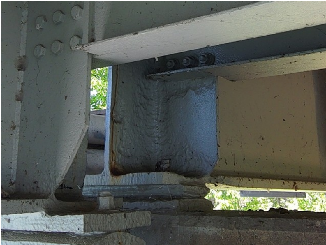
Span 10 Beam 1: 10 INCH LONG X 12 INCH HIGH AREA OF 1/8 INCH SECTION LOSS (3/8 INCH REMAINING) WITH NO RUST ON RIGHT STIFFENER AT BENT 9 (PAR)
