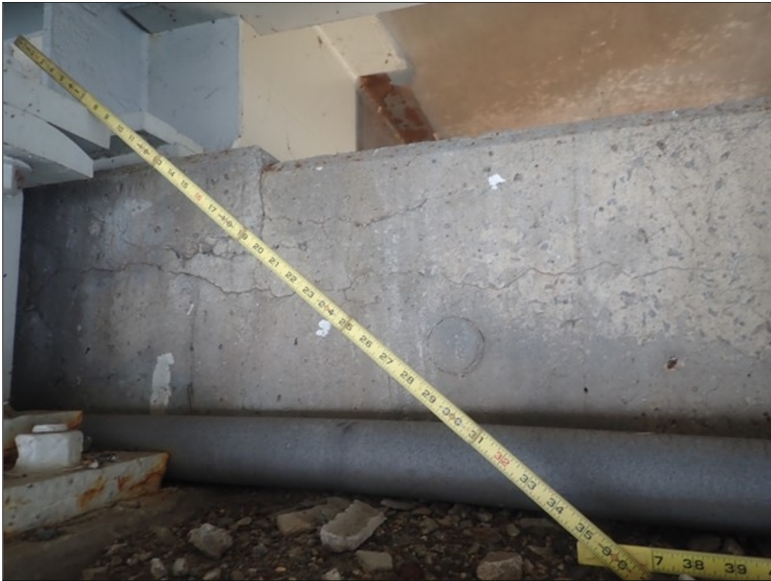
Bent 9 Cap 1: 18 INCHES LONG X 4 INCHES WIDE AREA OF DELAMINATION WITH 3 FEET LONG UP TO 1/16 INCH HORIZONTAL CRACKS ON SPAN 9 FACE OF BEAM STEP-UP UNDER BAY 3
