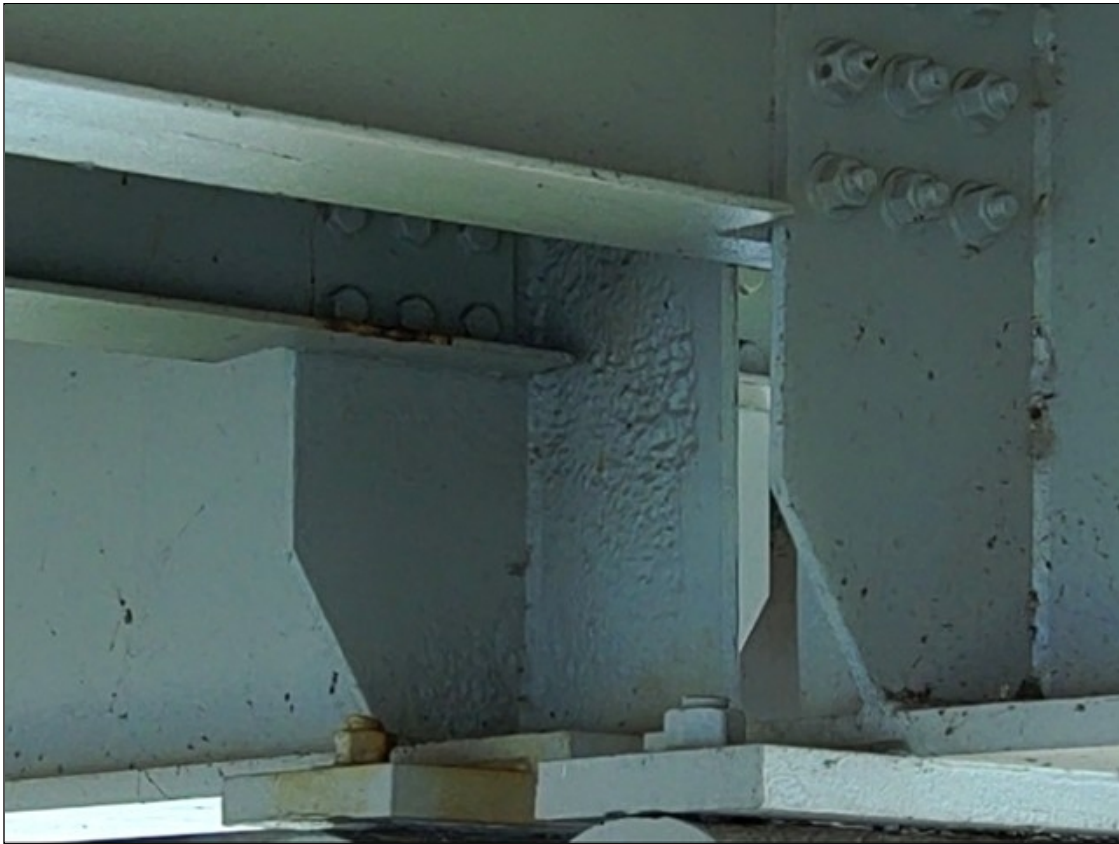
Span 2 Beam 3: 9 INCHES LONG X 24 INCHES HIGH AREA OF 1/4 INCHES SECTION LOSS (1/2 INCHES REMAINING) ON WEB IN SPAN 5 AT BENT 5 (CLEANED AND PAINTED) (PAR)
