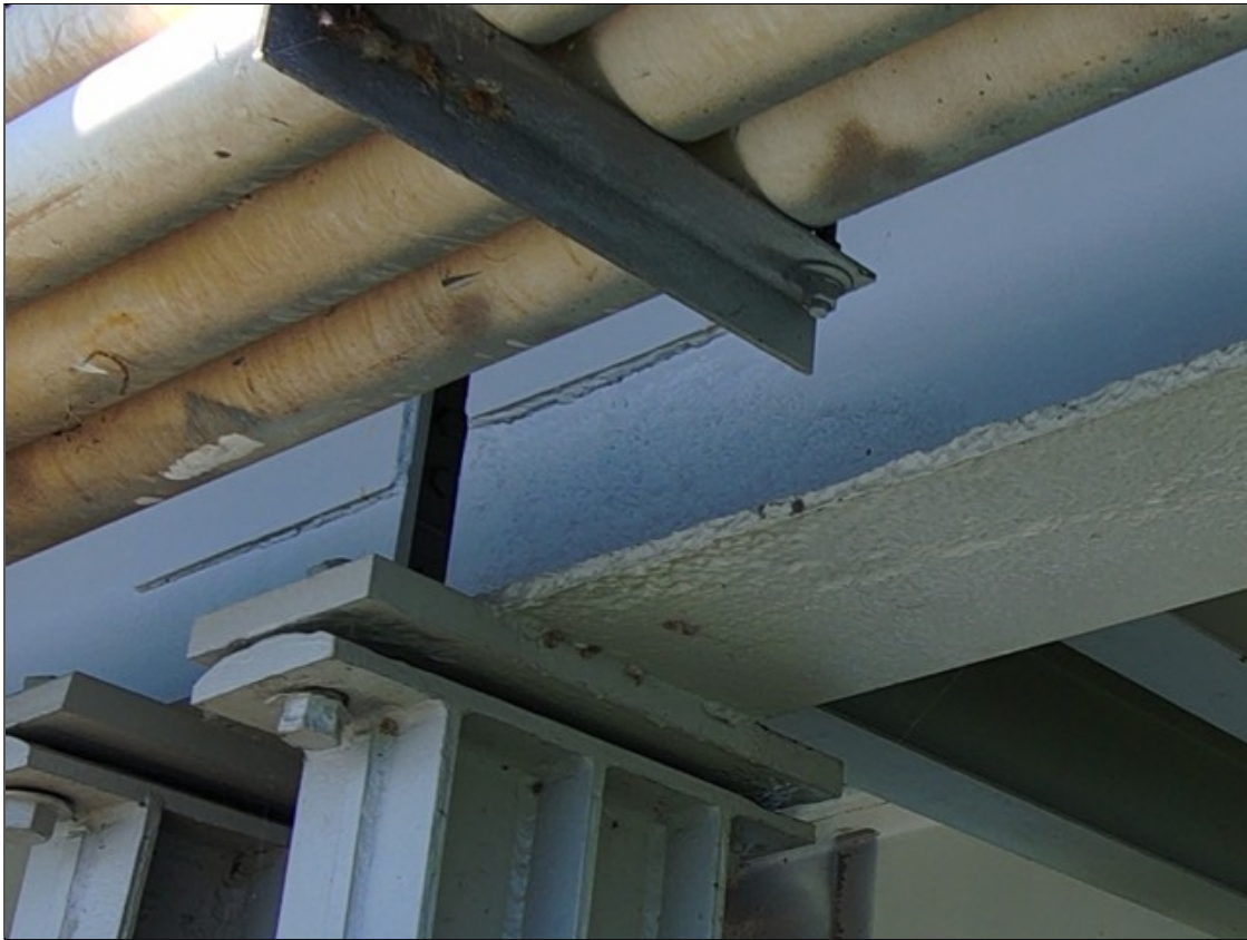
Span 2 Beam 1: 5 INCHES LONG X 11 INCHES HIGH AREA OF 1/8 INCH SECTION LOSS (3/8 INCH REMAINING) WITH NO RUST ON BOTH SIDES OF WEB AT BENT 5 (PAR) (CLEANED AND PAINTED)
